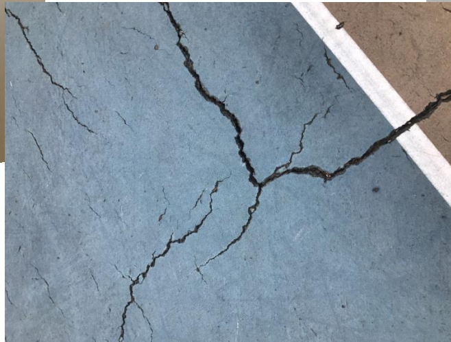
Cracked Tennis courts
