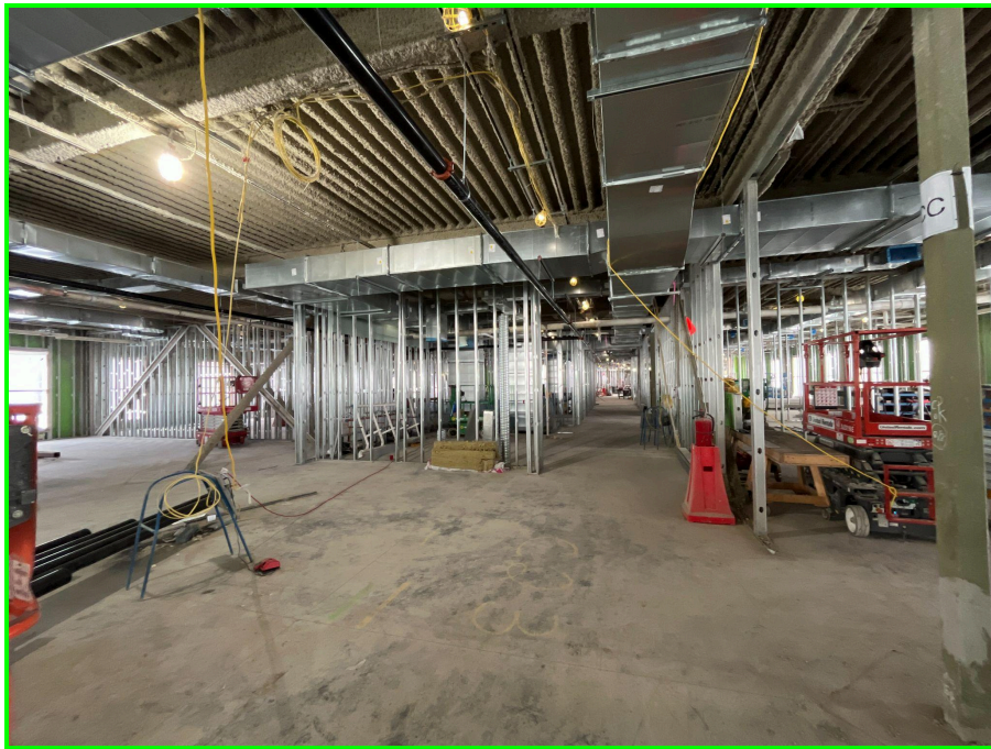
Inside the right wing, looking toward the center and left wings, framing work is underway and the mechanical, electrical, and plumbing rough-ins are advancing.
