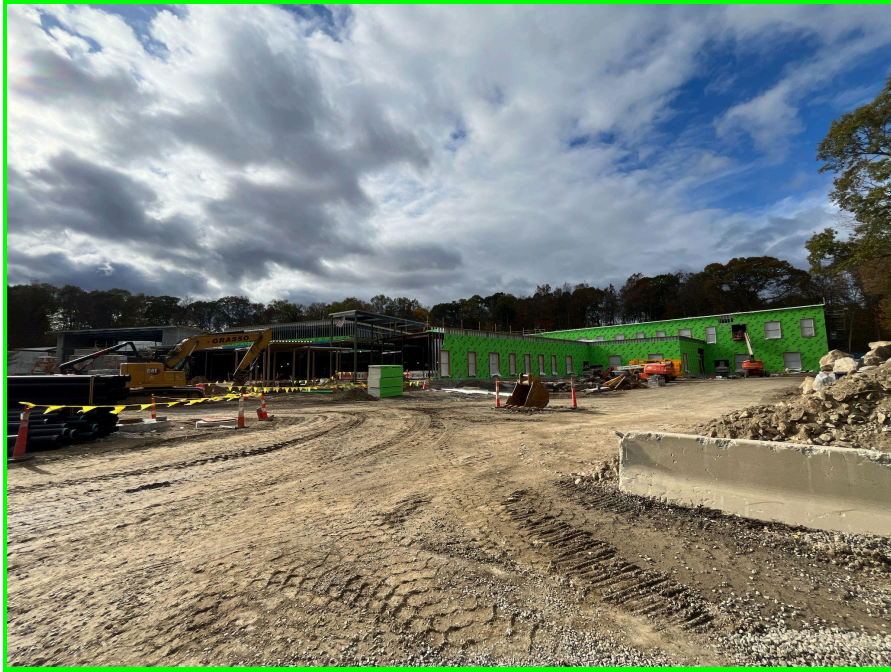
Outside the building, the structural steel and exterior sheathing are progressing to enclose the building.
