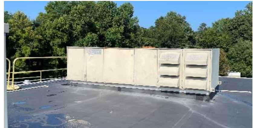
Rooftop units serving the cafeteria.
