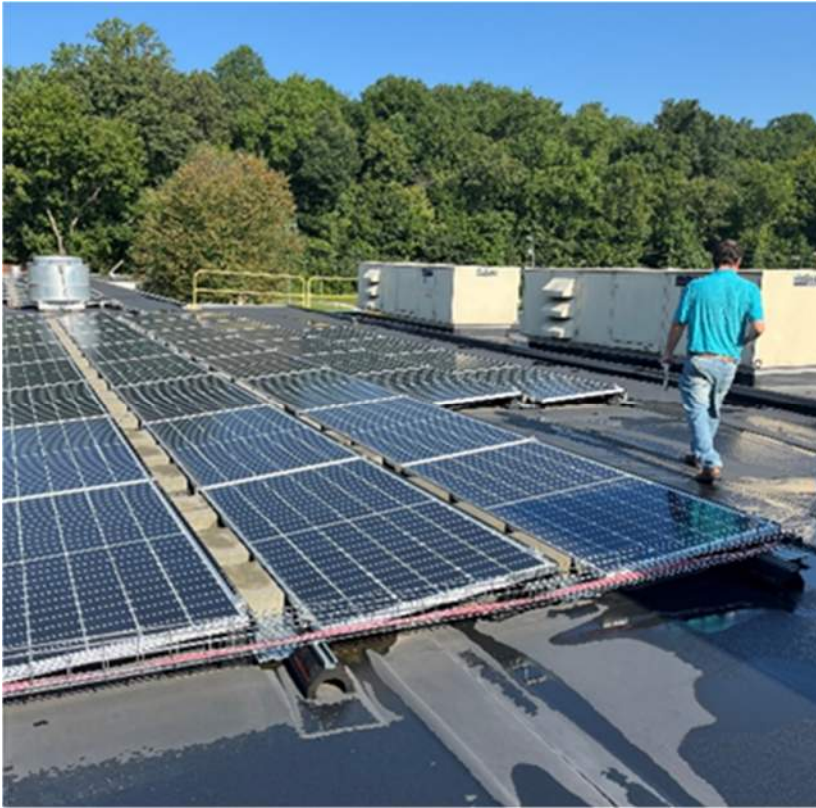
Roof top photovoltaic system.
