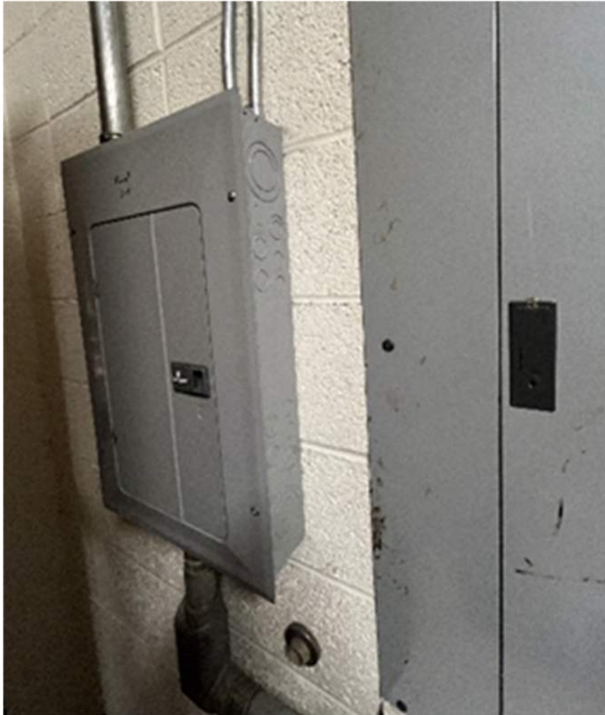
Electrical Distribution in MDF Room
