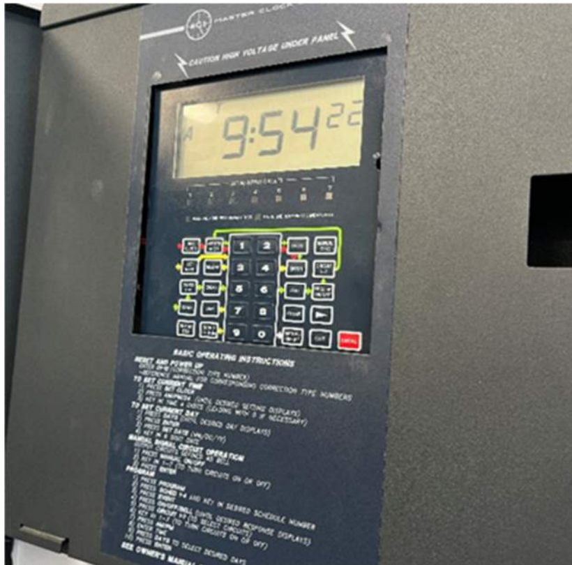
Notifier clock system in the Administration Suite.
