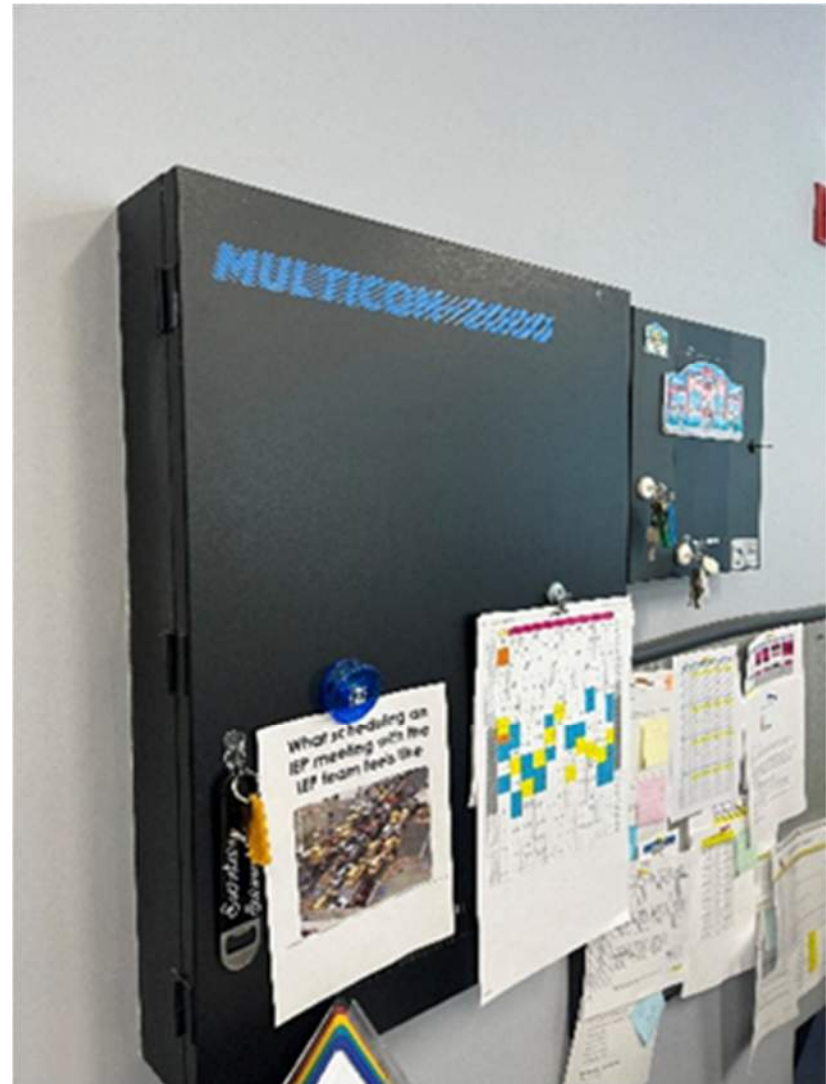
Multicom PA System in the Administration Suite
