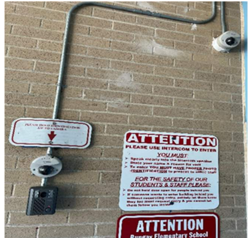
Security camera at the Building Main Entrance
