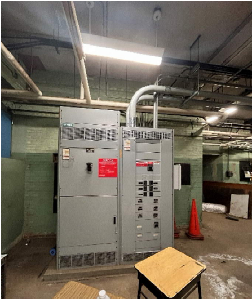
Main switchboard in basement boiler room.
