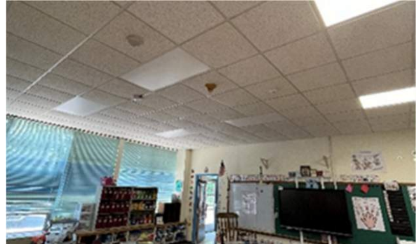
Typical Classroom Lighting
