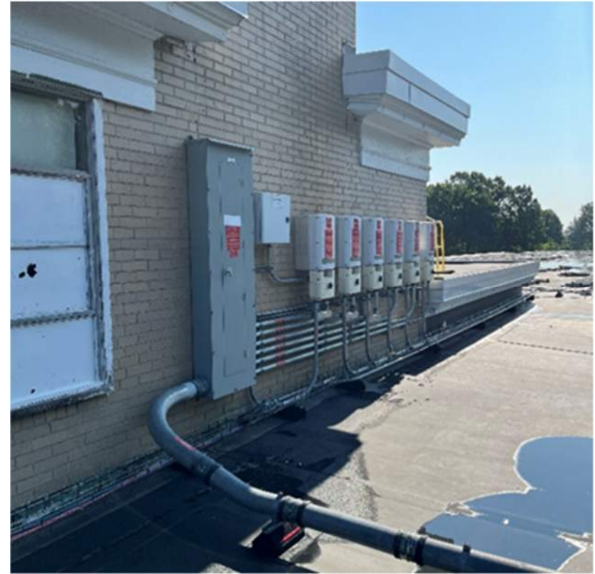
Roof top 480V Solar Equipment.
