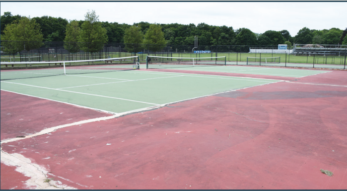
The high school tennis courts, also used by community residents, are cracked and in disrepair, creating a safety issue.
