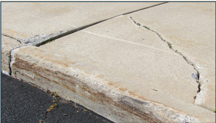
Cracked curbing and siding present safety issues for our students and staff.
