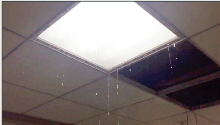
Roofs at all four schools leak when it rains.
