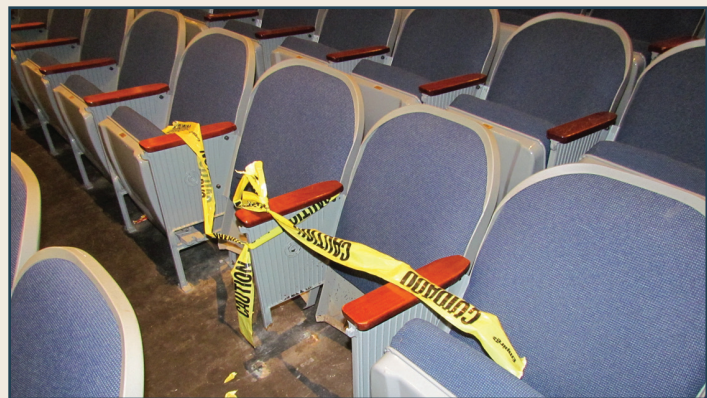
Broken seating and torn carpets would be replaced through auditorium renovations at the middle and high schools.
