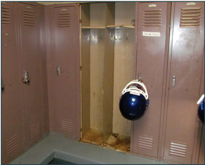
The locker rooms at Elwood Middle School, original to the building's construction, are in disrepair.
