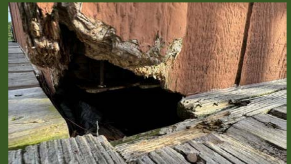
Deteriorated Exterior Trim
