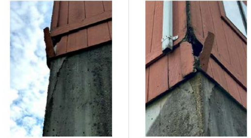
Vertical cracks in the foundation
