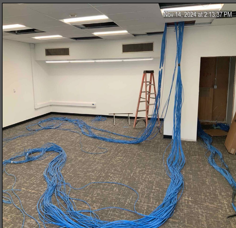
November 2024 – Network Cabling
