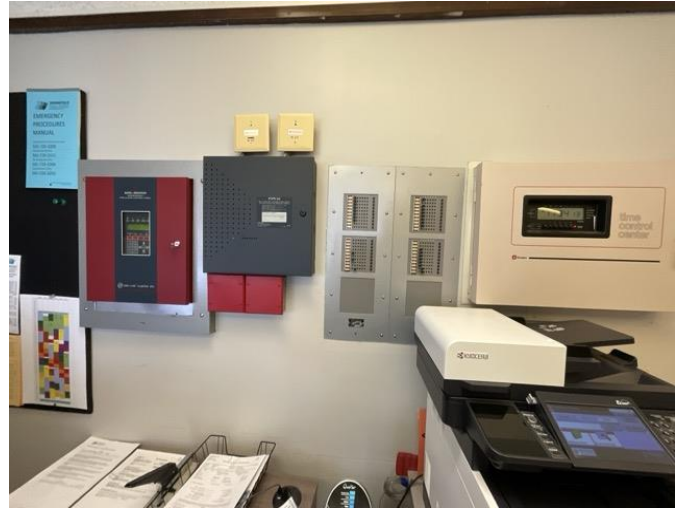
2 - FIRE ALARM PANEL
