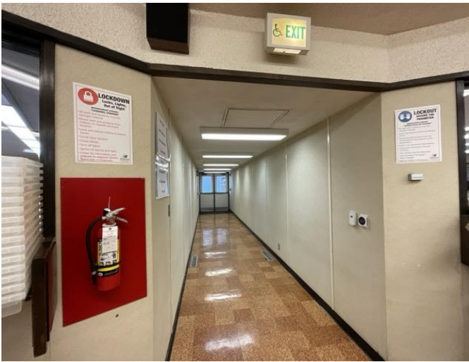
11 - FIRE ALARM SYSTEM
