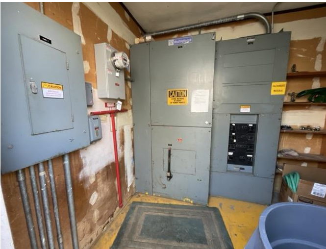
19 - MAIN ELECTRICAL ROOM
