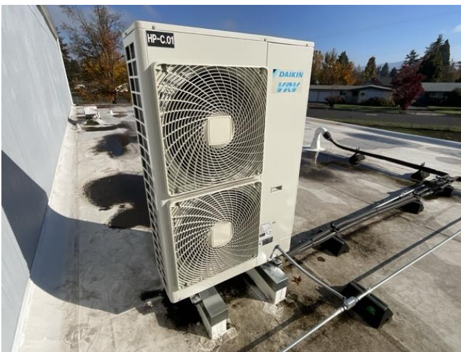
9 - VRV HEAT PUMPS UNITS
