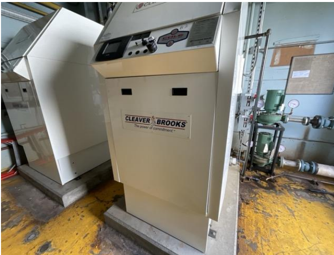
13 - BOILERS AND PUMPS
