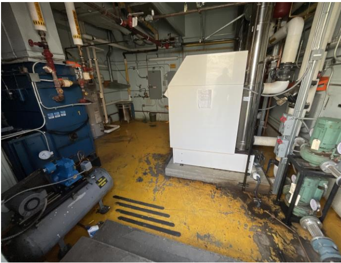
5 - MAIN MECHANICAL ROOM
