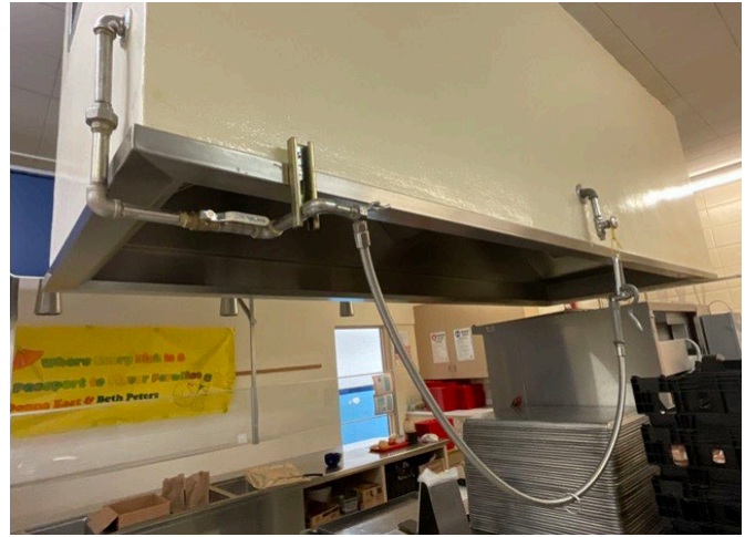
20 – FIRE SUPPRESSION SYSTEM
