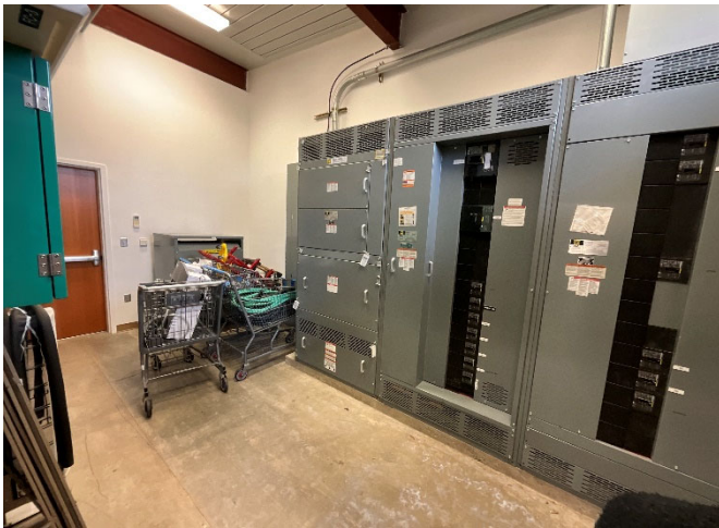
15 – MAIN ELECTRICAL ROOM
