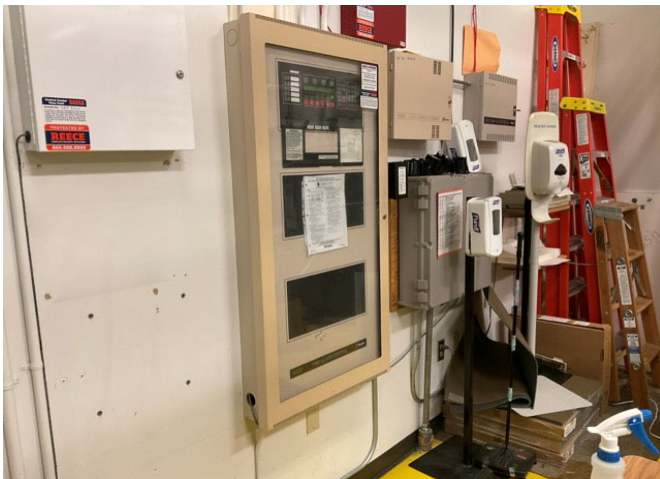
23 – FIRE ALARM PANEL
