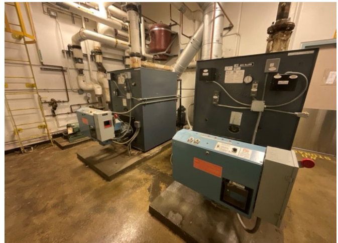
20 – BOILERS AND PUMPS
