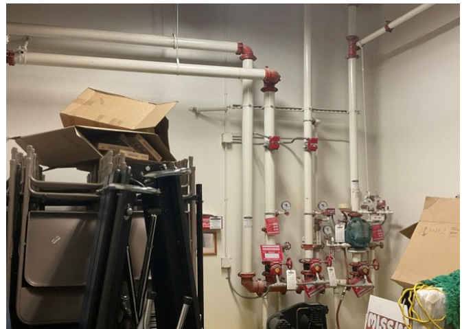
24 – FIRE SPRINKLER RISERS
