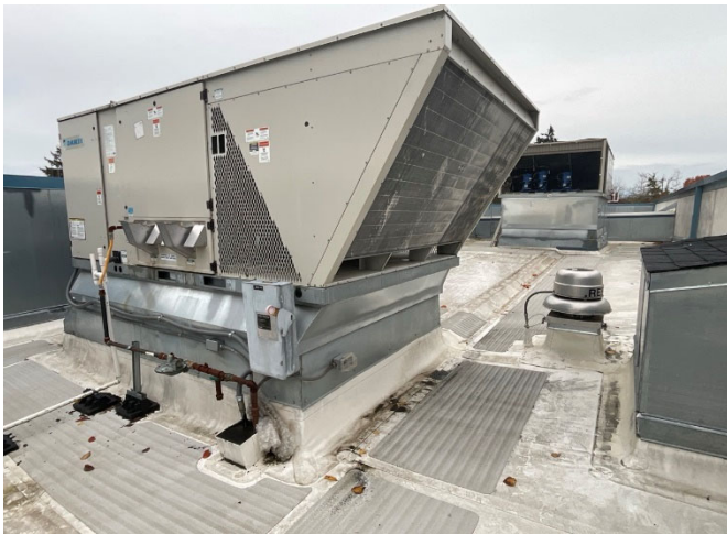
19 – ROOFTOP MECHANICAL EQ
