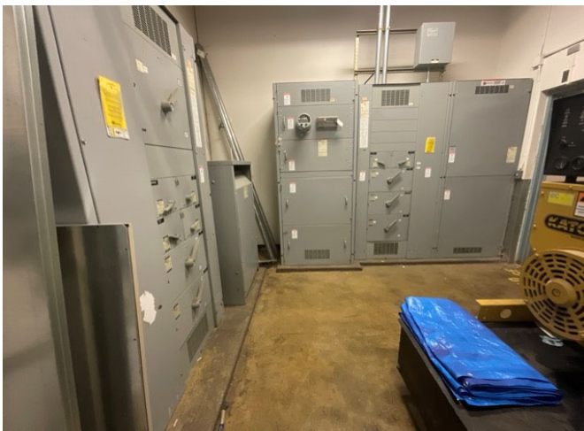
21 – MAIN ELECTRICAL ROOM
