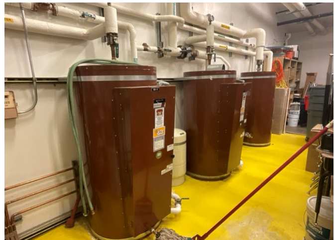
18 – DOMESTIC HOT WATER SUPPLY
