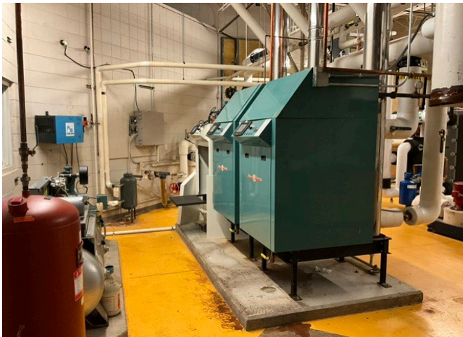
23 – BOILERS AND PUMPS
