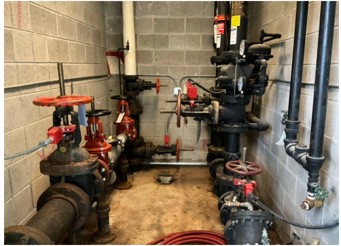
26 – FIRE SPRINKLER RISERS
