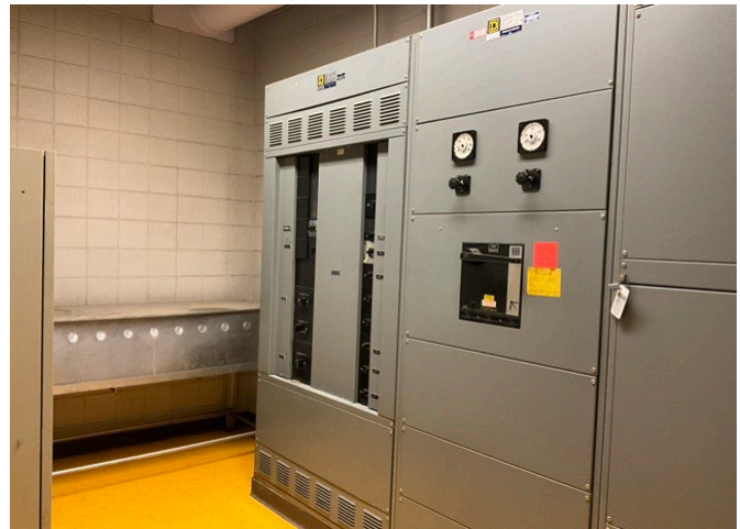
24 – MAIN ELECTRICAL ROOM
