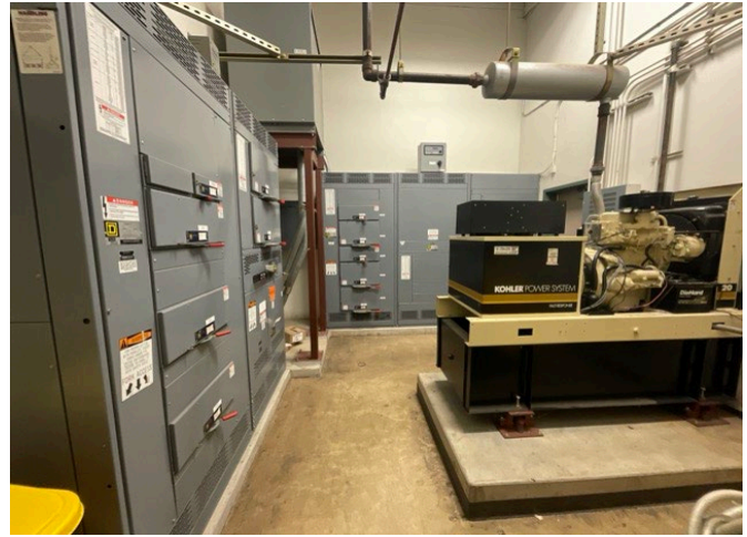
26 – MAIN ELECTRICAL ROOM
