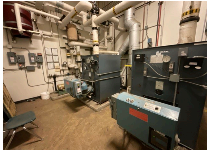
20 – BOILERS &amp; PUMPS
