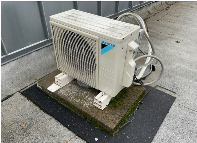
23 – SPLIT SYSTEM DUCTLESS
