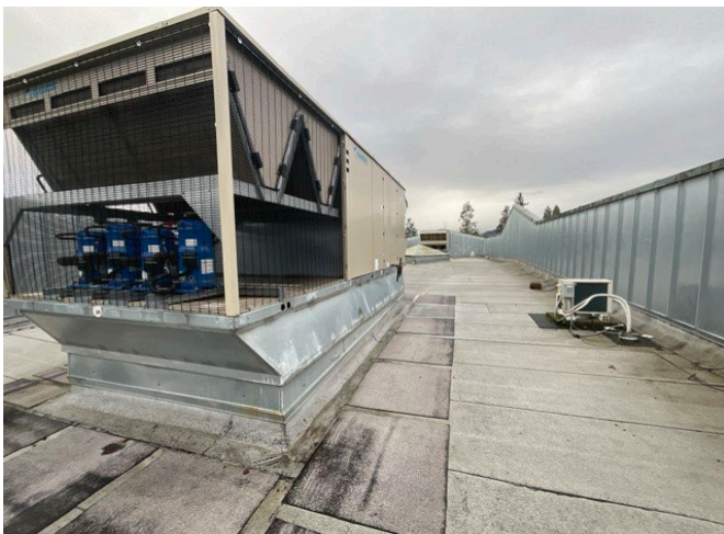
21 – ROOFTOP MECHANICAL EQUIPMENT
