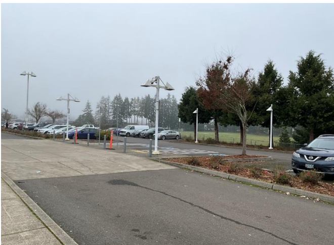
3 – POLE LIGHT FIXTURE WITH LAMPS
