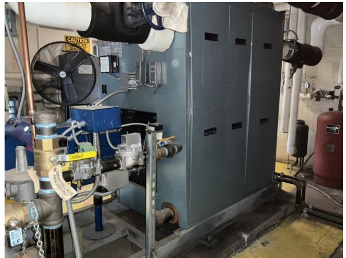
14 - BOILERS AND PUMPS
