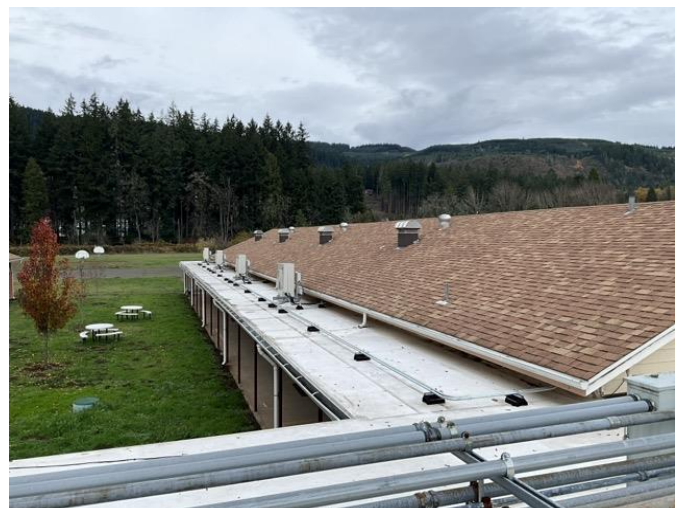
16 - ROOFTOP MECHANICAL EQUIPMENT
