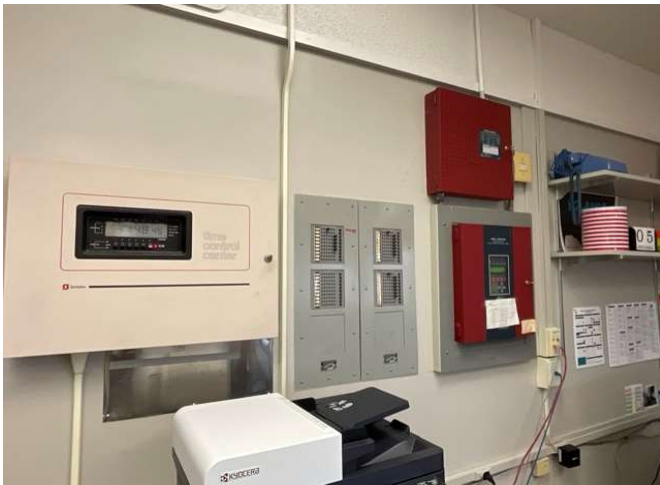
13 – FIRE ALARM PANEL
