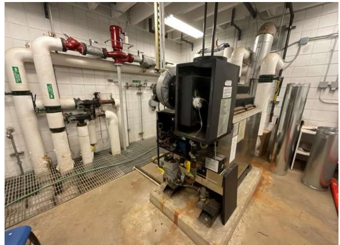
10 – HVAC BOILERS &amp; PUMPS
