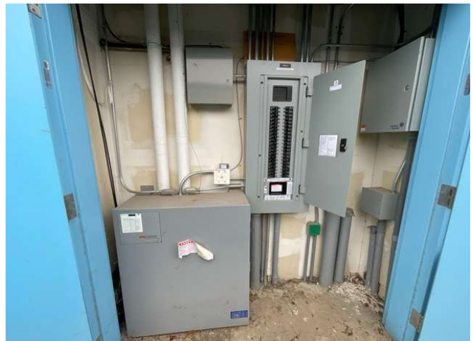
6 – MAIN ELECTRICAL PANEL
