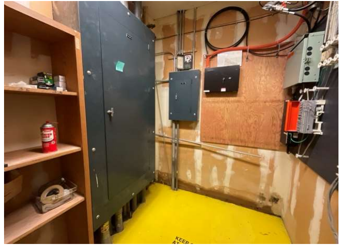
2 – MAIN ELECTRICAL PANEL
