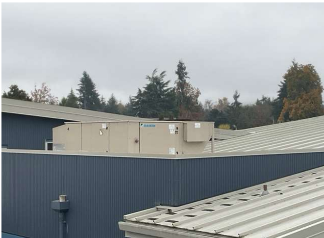
5 – ROOF HVAC UNIT
