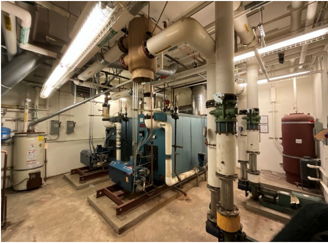
13 – MAIN MECHANICAL ROOM
