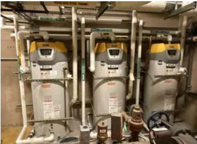
17 - DOMESTIC HOT WATER SUPPLY
