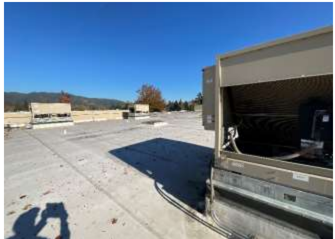
18 - ROOFTOP MECHANICAL EQ
