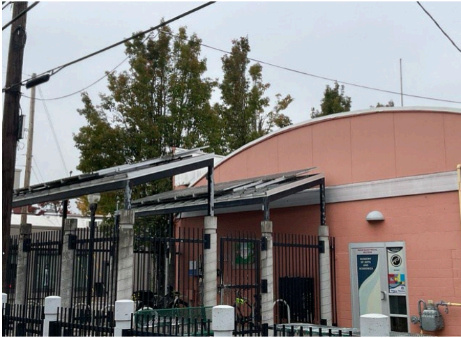
1 – SOLAR POWER PANELS
