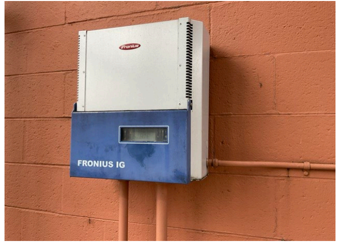
2 – SOLAR POWER INVERTER
