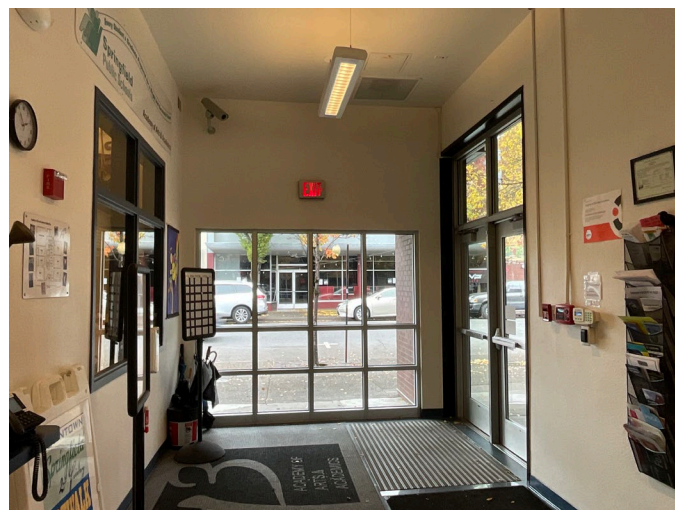
24 - FIRE ALARM SYSTEM
