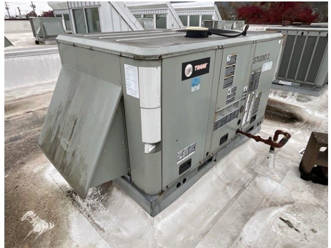
20 - ROOF MOUNTED PACKAGED UNIT
