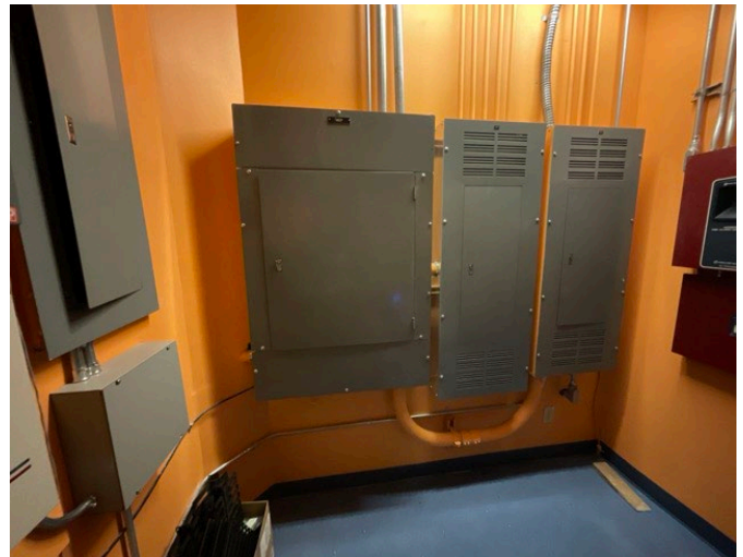
22 - MAIN ELECTRICAL ROOM
