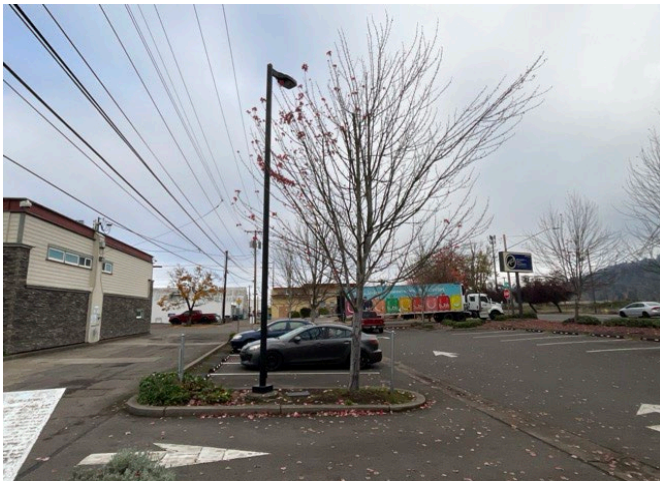
11 – POLE LIGHT FIXTURE WITH LAMPS
