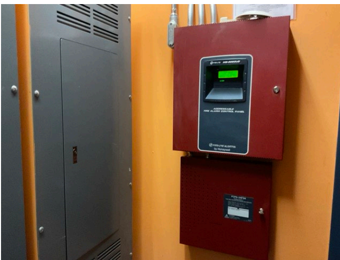
23 - FIRE ALARM PANEL
