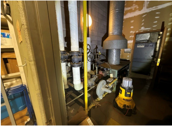
13 – MAIN MECHANICAL ROOM
