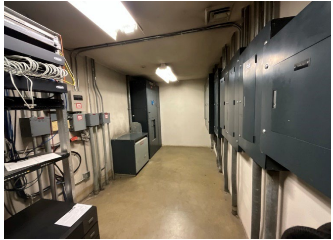
14 – MAIN ELECTRICAL ROOM
