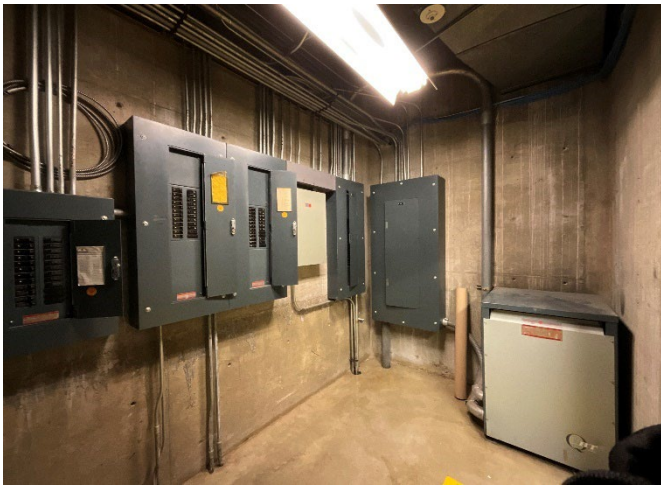
9 – MAIN ELECTRICAL ROOM
