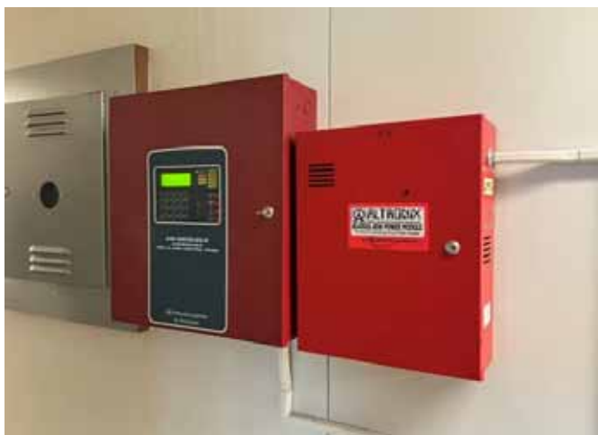
23 – FIRE ALARM PANEL
