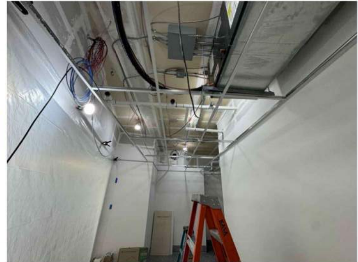
PR08 Overhead MEP & Ceiling Grid
