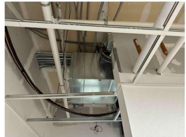
PR08 Overhead MEP in Kitchen
