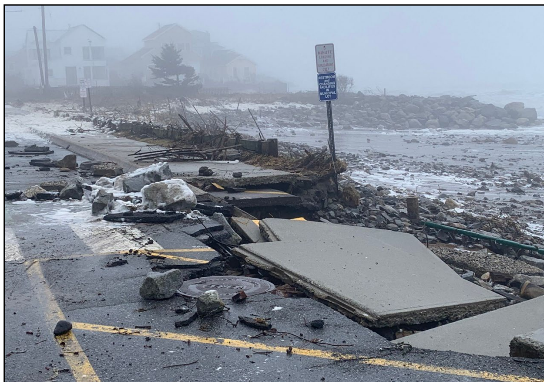
Figure 2-1. Damage Along Bayview Avenue after January 2024 Storms
