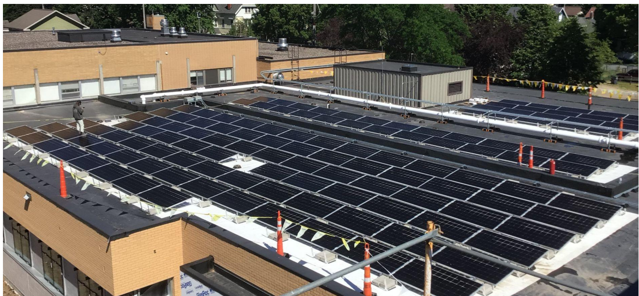
Figure 9. Solar panels on top of Hamilton Elementary School.
