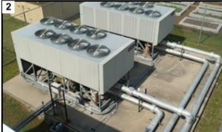
Trane air cooled chillers
