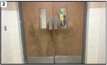
Fine Arts - Replace aged doors and frame.
