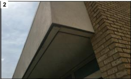
Replace metal soffit trim and wood blocking, typical. Repair cracks in plaster veneer.
