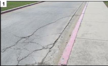
Failed Concrete Pavement - Removed and Replace Subgrade and Concrete
