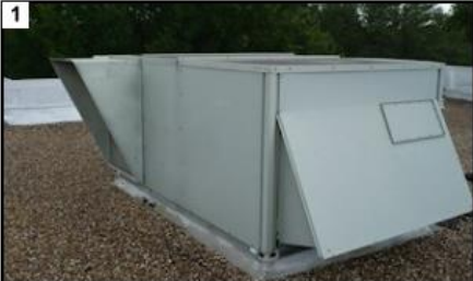
Trane rooftop a/c unit
