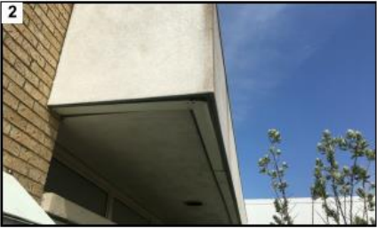
Replace metal soffit trim and wood blocking, typical. Repair cracks in plaster veneer.
