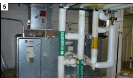
Lower level Trane VAV air handling unit
