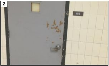
Fine Arts - Replace aged doors and frame.
