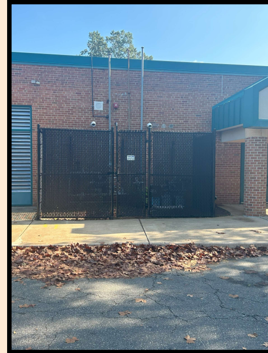
Gas Meter Fencing
