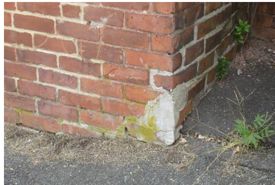
Brickwork and mortar deterioration
