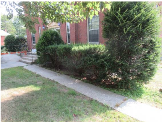
The overgrown vegetations should be kept clear of the building so surfaces will dry.
