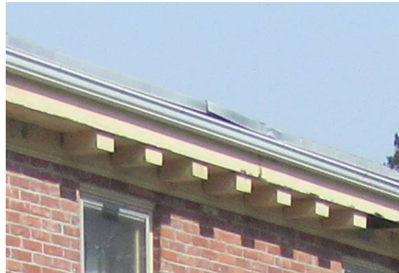
Damaged roof metal edge trim/fascia
