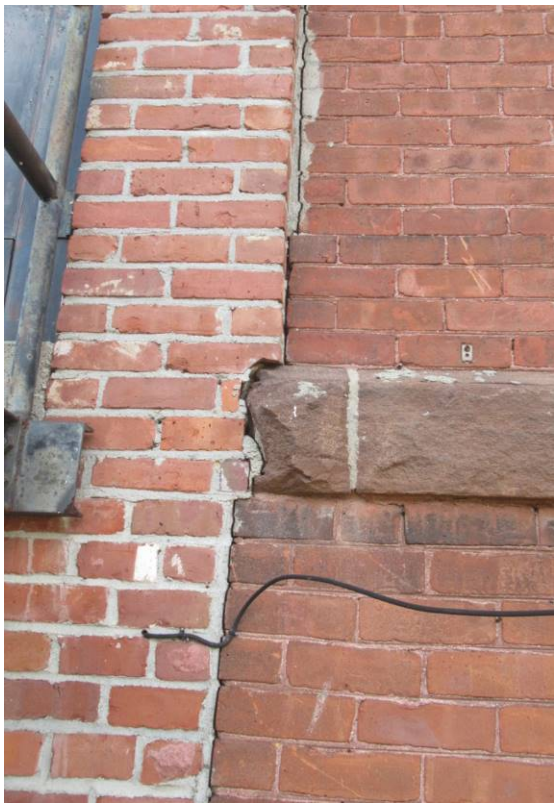
Seal joint between 1904 and 1960 buildings. (Irregular building settlement)
