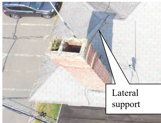
Remove vegetation (Review lateral supports for chimneys. Paint supports to retard rust and staining.)
