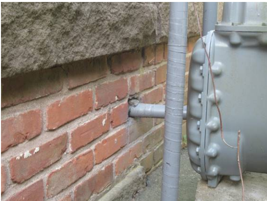
Wall penetrations should be sealed.
