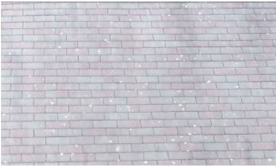
Lichen growth on the northerly and westerly roof slopes. (Little concern.)
