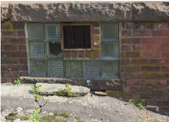
Broken glass blocks should be replaced or the entire window assembly replaced.
