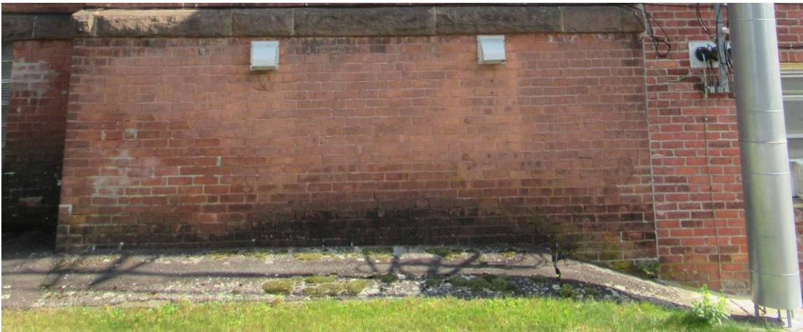
Moisture damage and algae growth on base of wall
