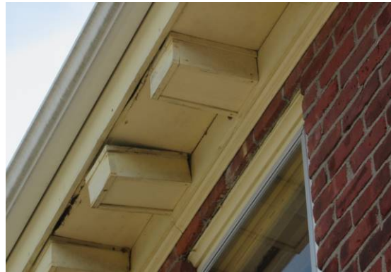
Repair/replace rotted/damaged woodwork.
