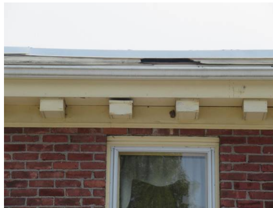
Repair/replace rotted/damaged woodwork.
