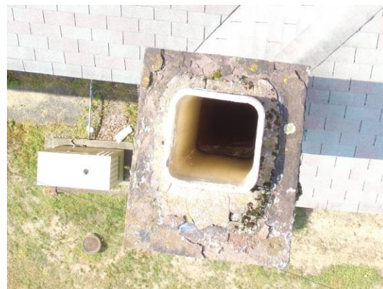
Deteriorated masonry around chimney cap.
