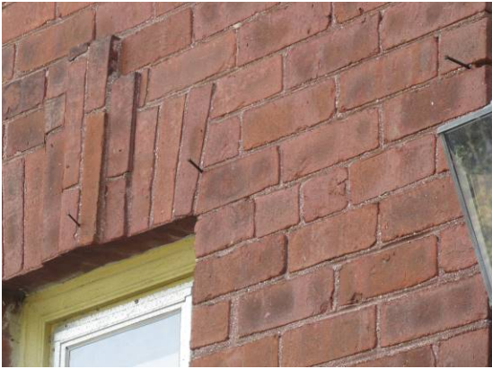
Miscellaneous projecting items (nails) should be removed and the grout joints repaired.
