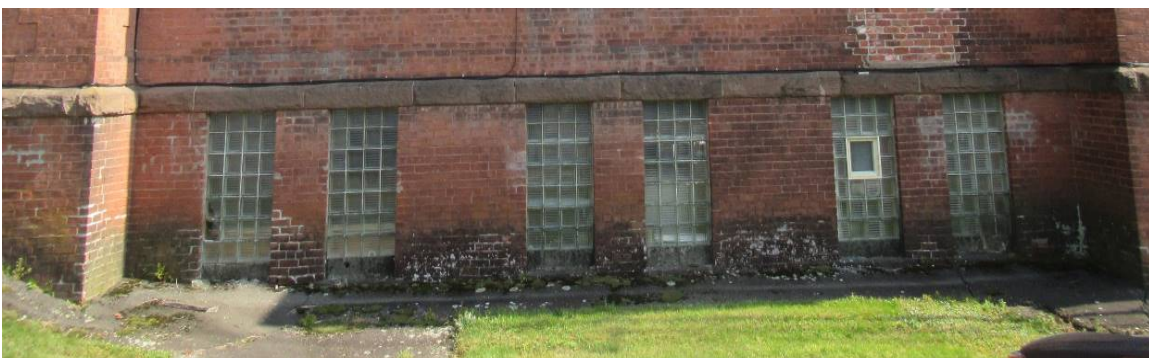
Moisture damage and algae growth on base of wall
