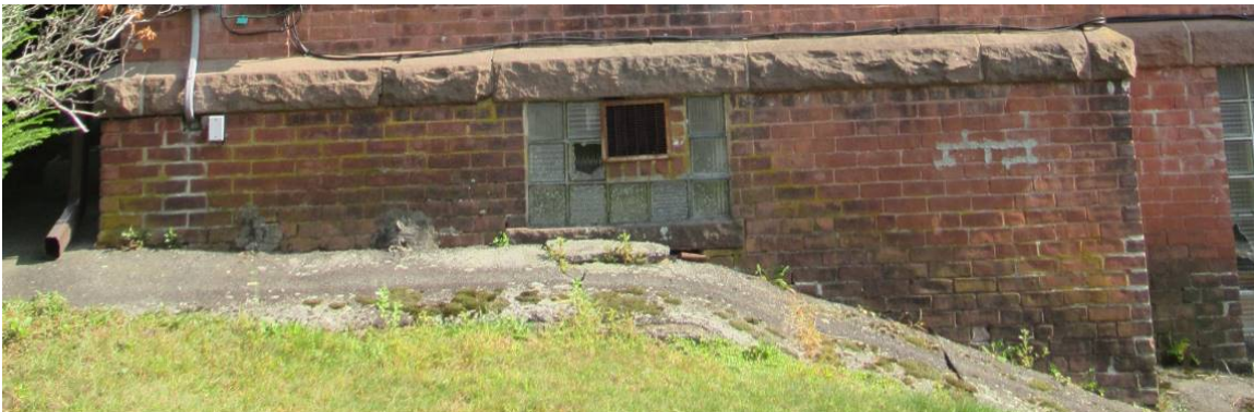
Moisture damage and algae growth on base of wall
