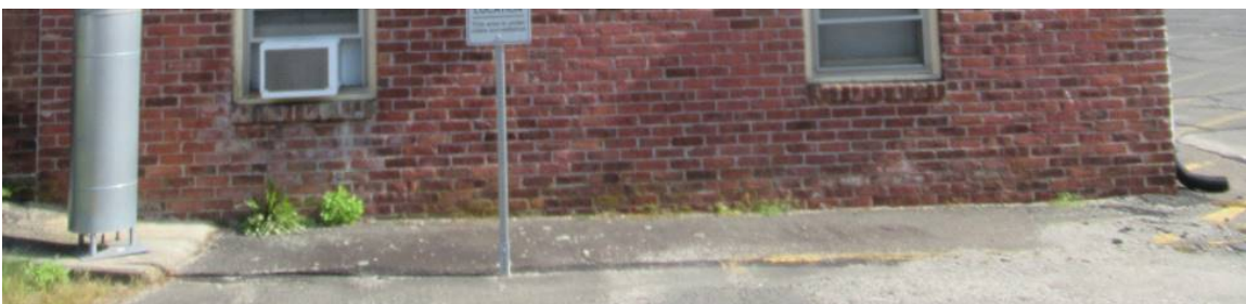
Moisture damage and algae growth on base of wall (1960 Addition)
