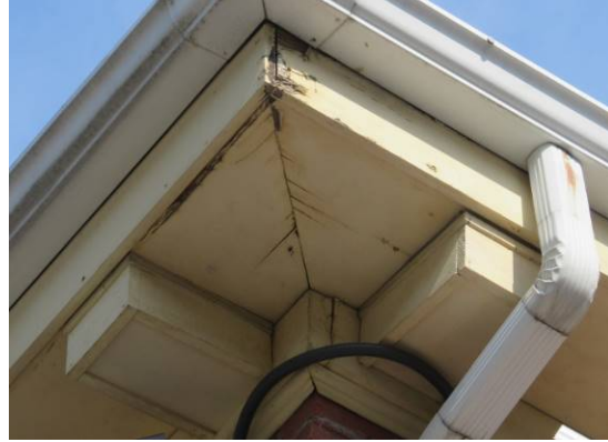
Repair/replace rotted/damaged woodwork.
