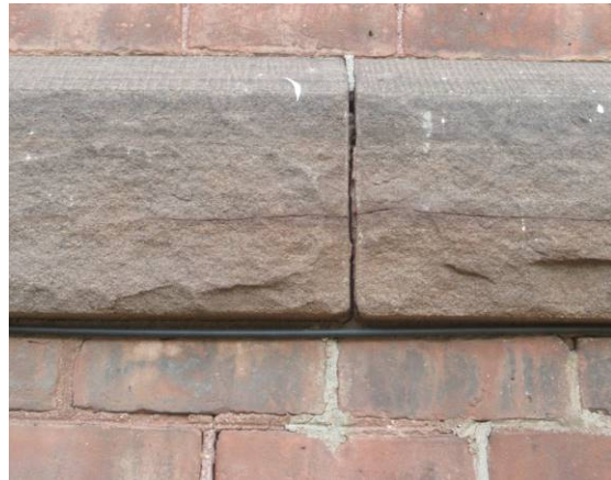
Mortar joint deterioration
