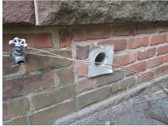
Wall penetrations should be weatherproof and vermin proof.
