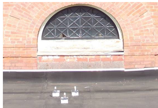
Abandoned antenna mounts (Remove with next roof replacement)
