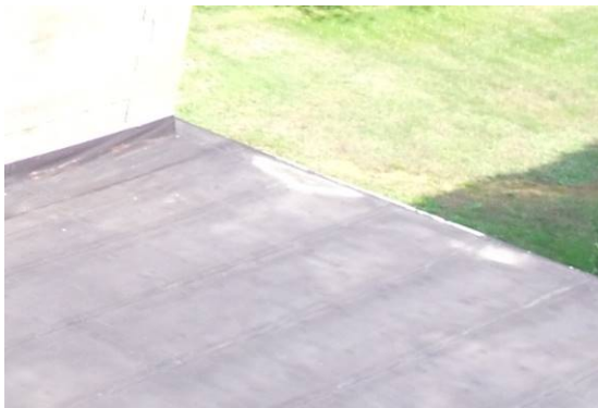
Minor evidence of debris/ponding (Research depression in insulation)
