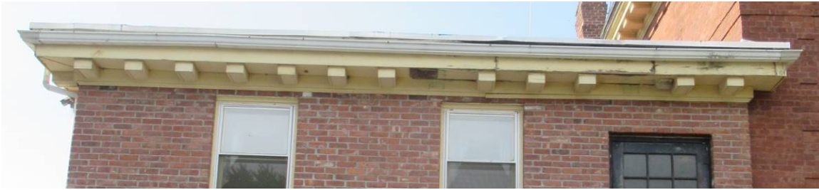
Repair/replace rotted/damaged woodwork.
