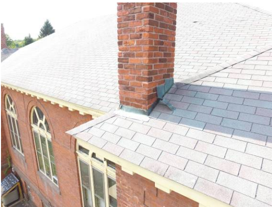
Step flashing at chimney requires repair.
