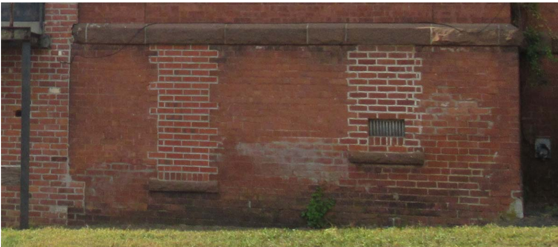
Moisture damage and algae growth on base of wall
