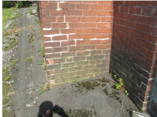
Brick damage and grout degradation
