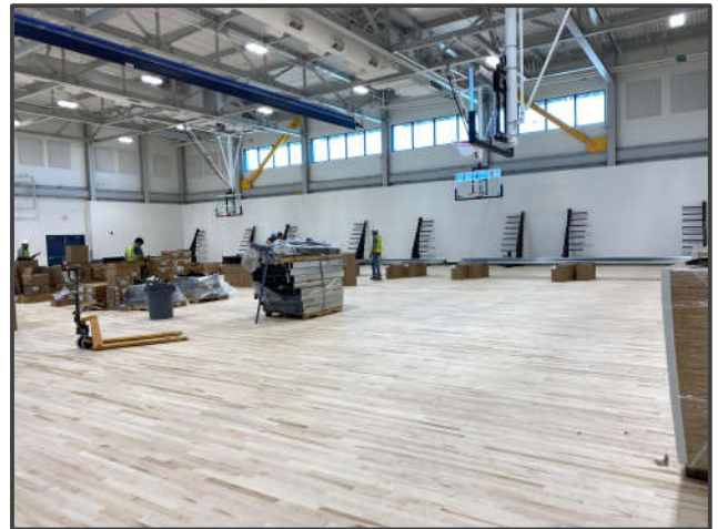
New Gym Building - Installation of bleachers while the floor is being finished
