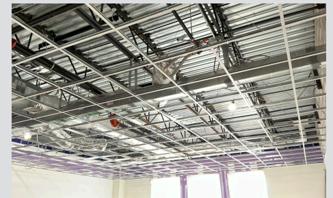
Ceiling grids are installed after Rough-In to support ceiling tiles, vents, and lights.
