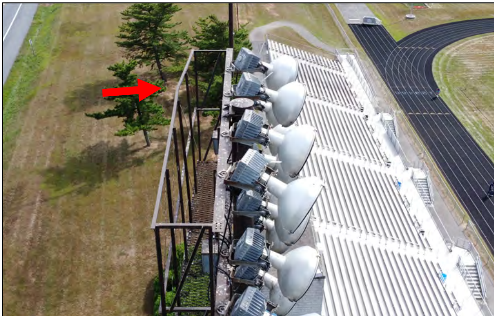
Pole NE1 Light Support Cage Condition
