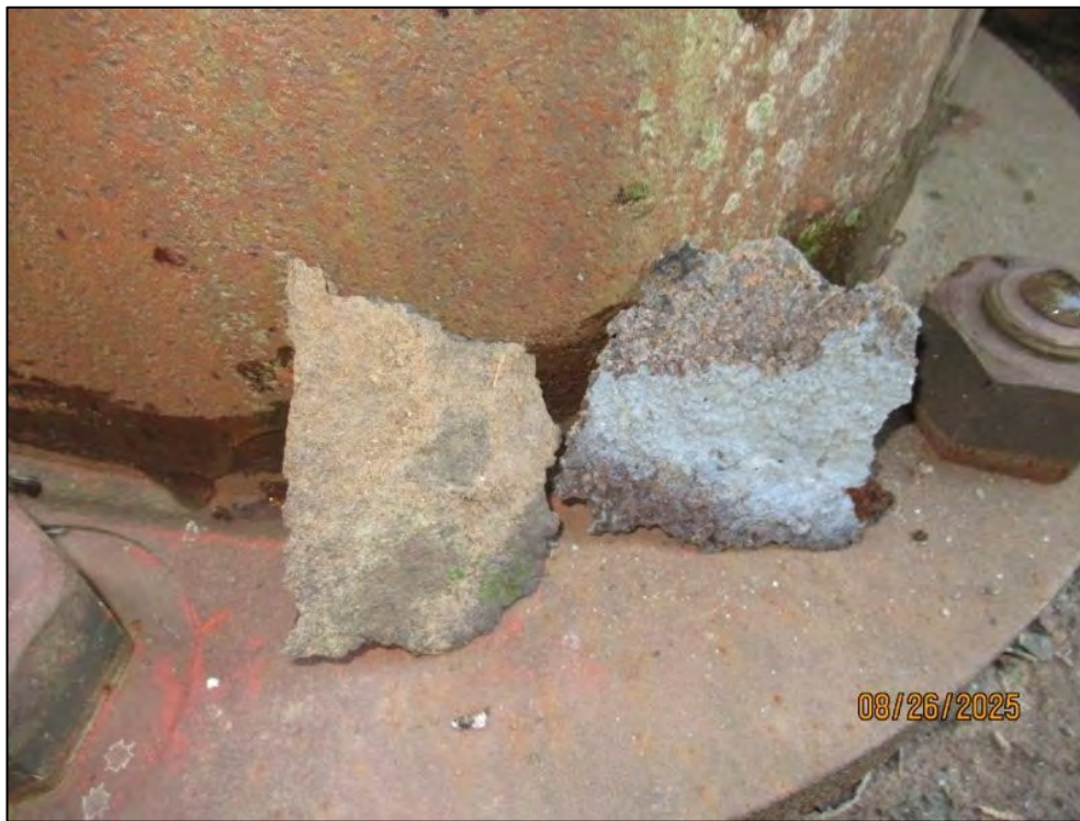
Pole NE1 Aggressive Interior Corrosion (Top) and Scaling Pole Base/Shaft Material
