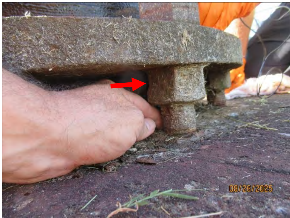
Pole SW3 Scaling Pole Material & Anchor Rod Material Loss of Threads and Hardware
