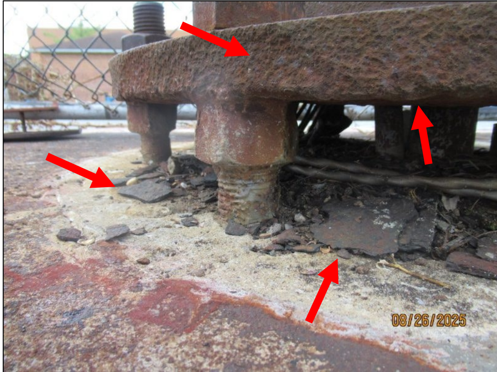
Deterioration of Pole S3 Base Plate and Scaling Pole Material Under the Base Plate
