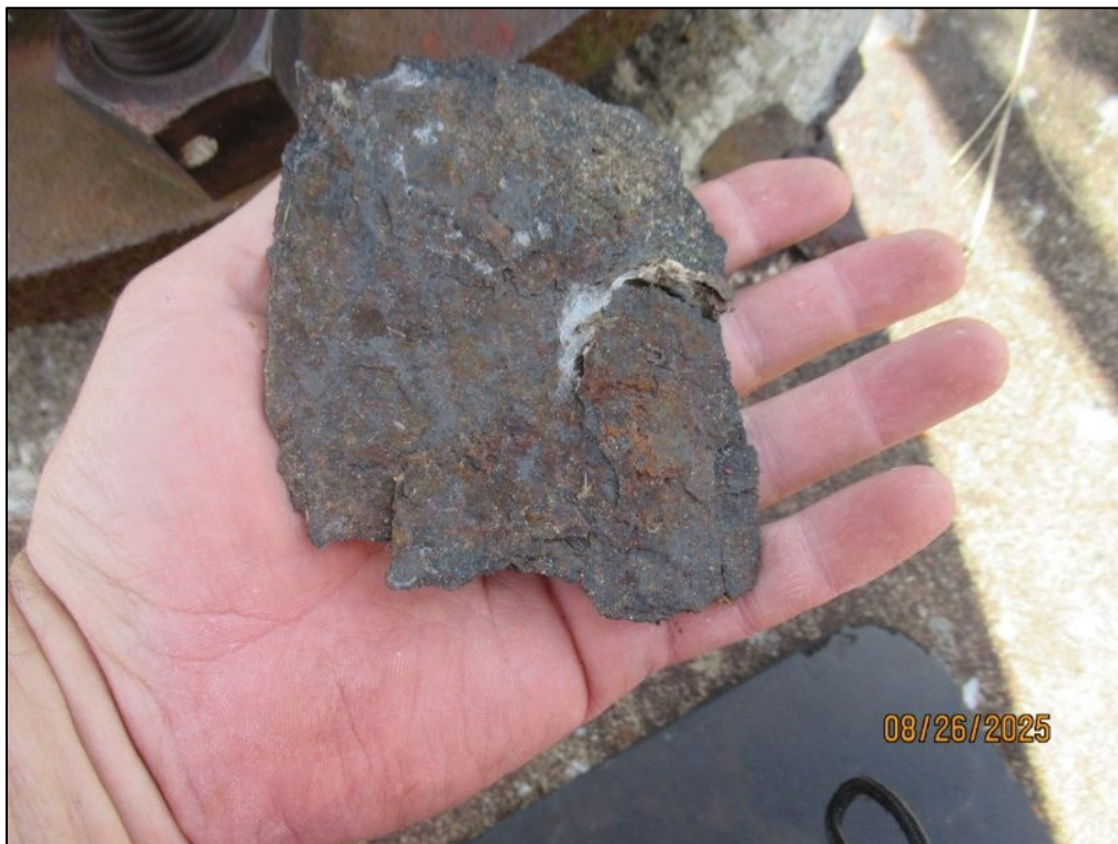
Pole S3 Aggressive Interior Corrosion (Top) and Scaling Pole Base/Shaft Material at Base
