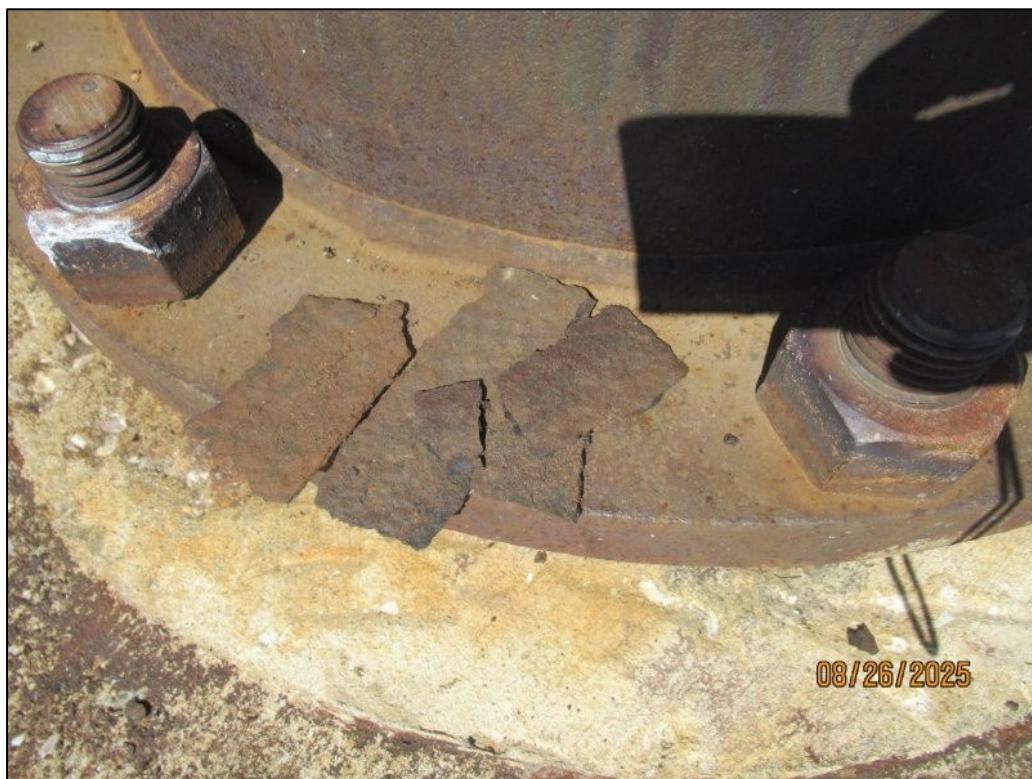
Deterioration of Pole W4 and Scaling Pole Material
