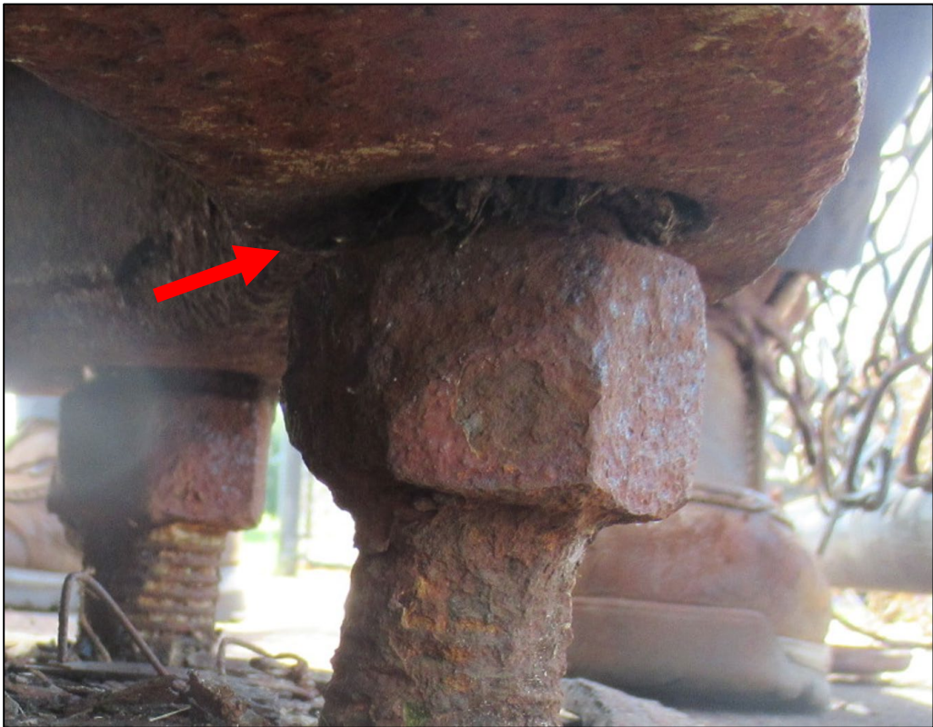
Pole S3 Anchor Rod Nuts Not in Contact With Base Plate
