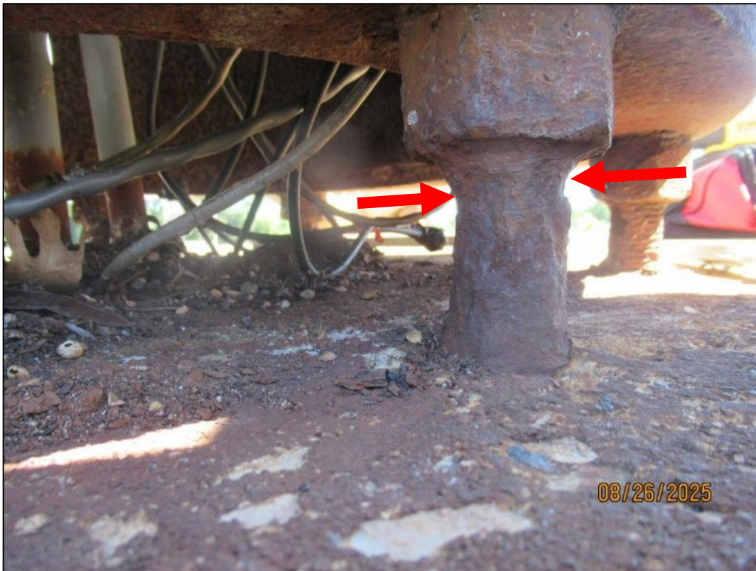
Pole W4 Anchor Rod Threads Missing and Reduction in Diameter from 1 1/2" to Approximately 1 1/8"
