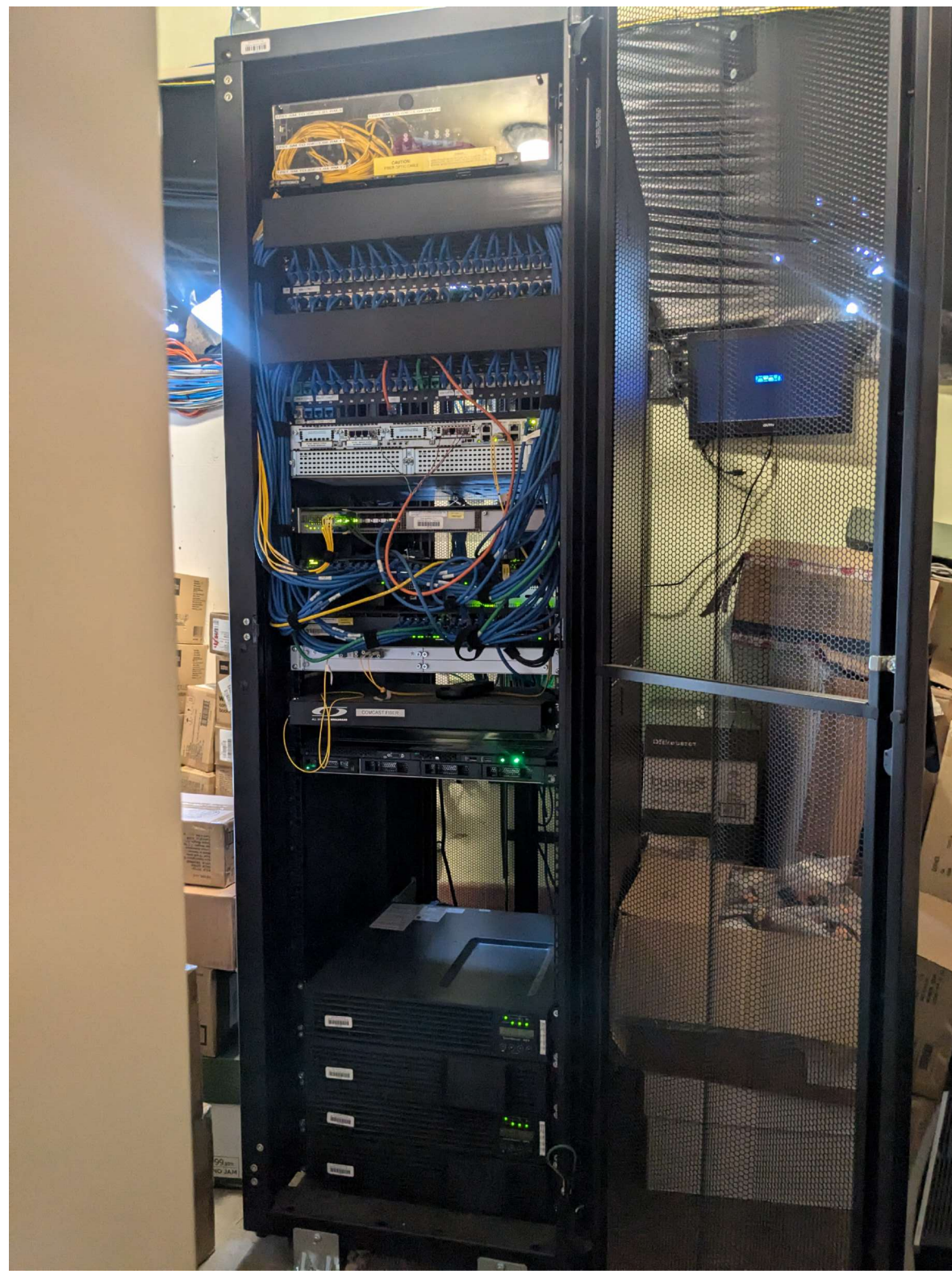
RACK - EXISTING CONDITION
