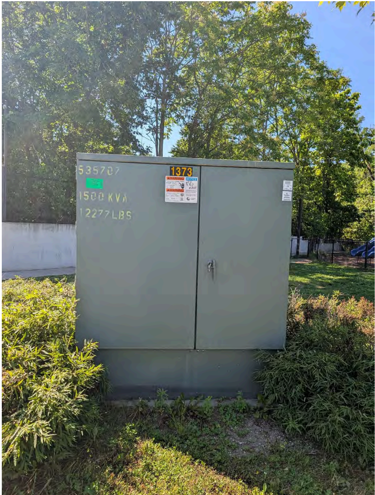
Exhibit 3.1 - Wendell Cross Photos of Existing Transformer
