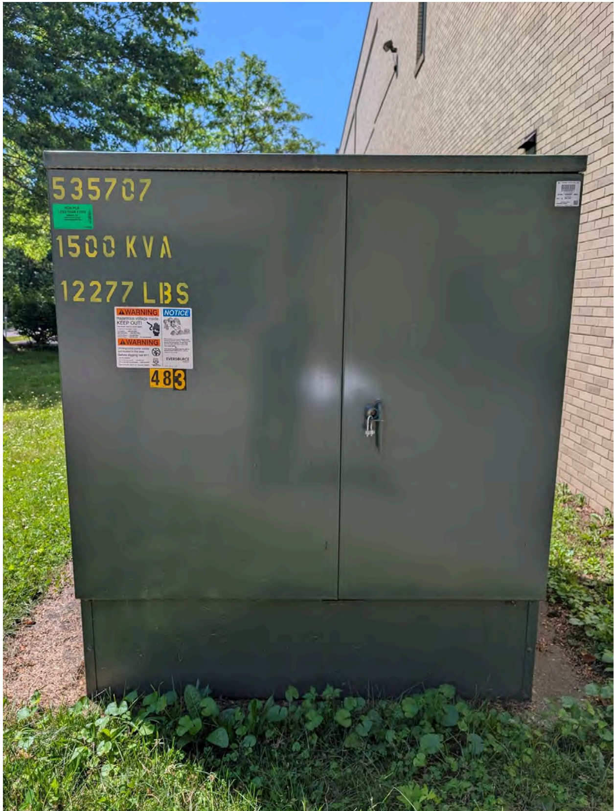
Exhibit 3.5 - West Side Middle School Photos of Existing Transformer
