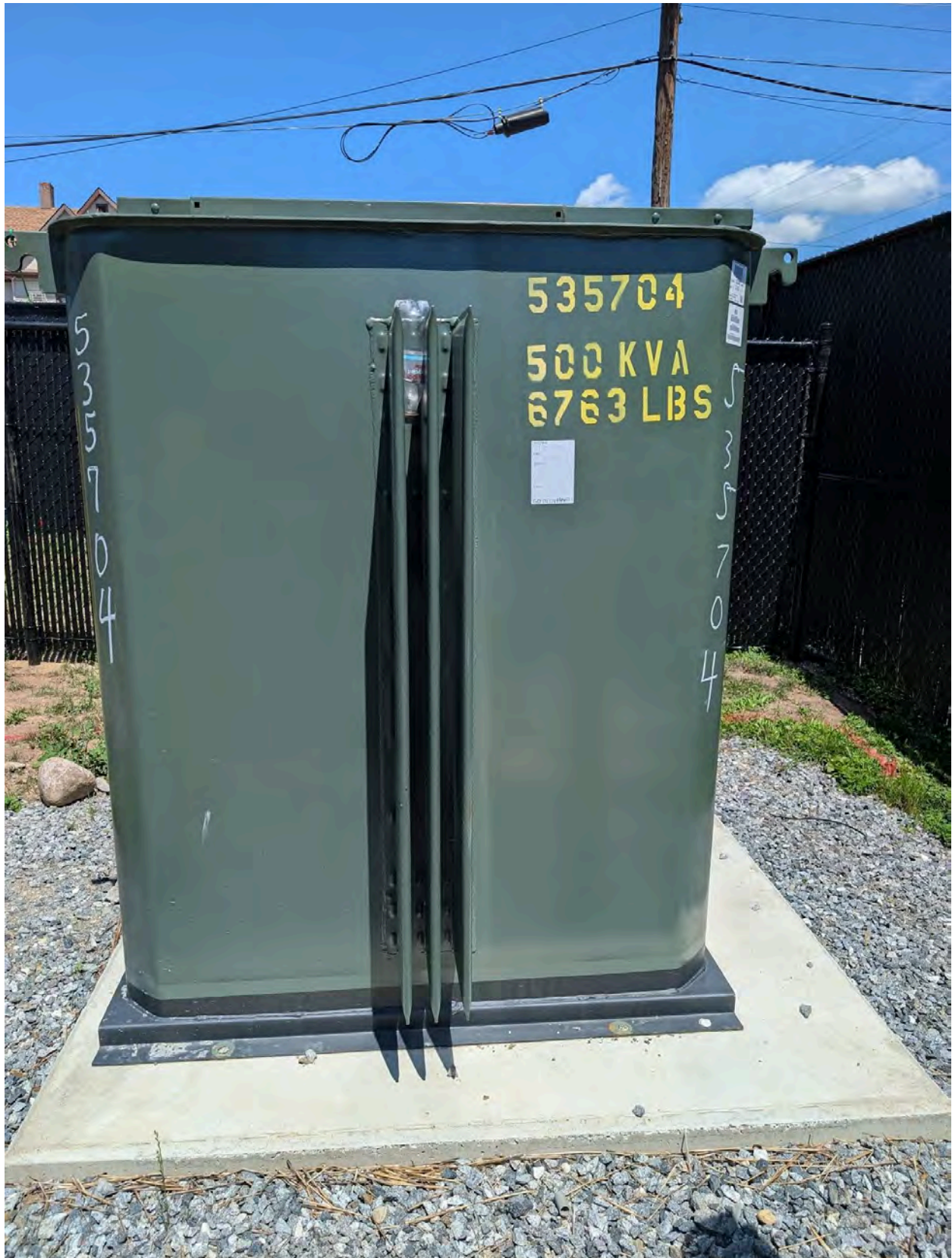
Exhibit 3.3 - Sprague Photos of Existing Transformer
