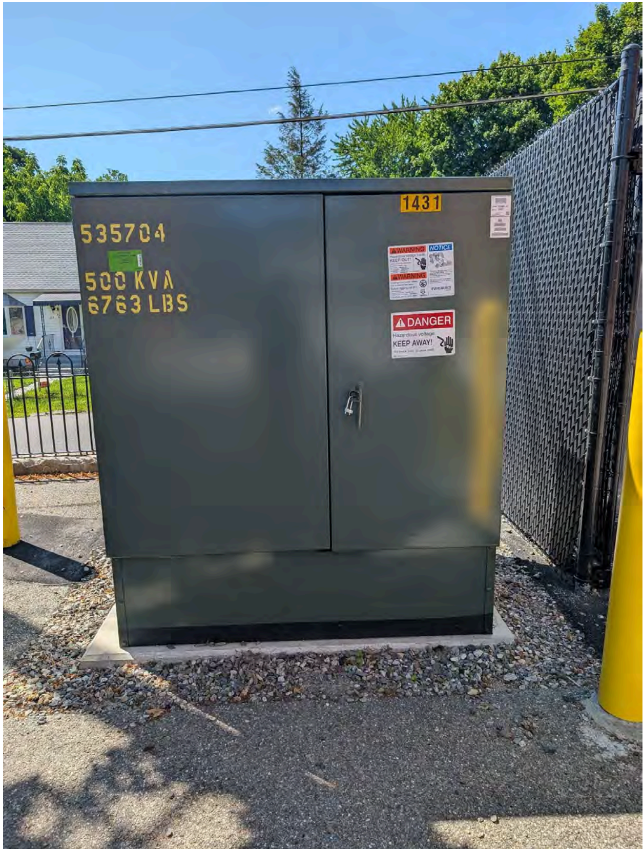
Exhibit 3.4 - B.W Tinker Photos of Existing Transformer
