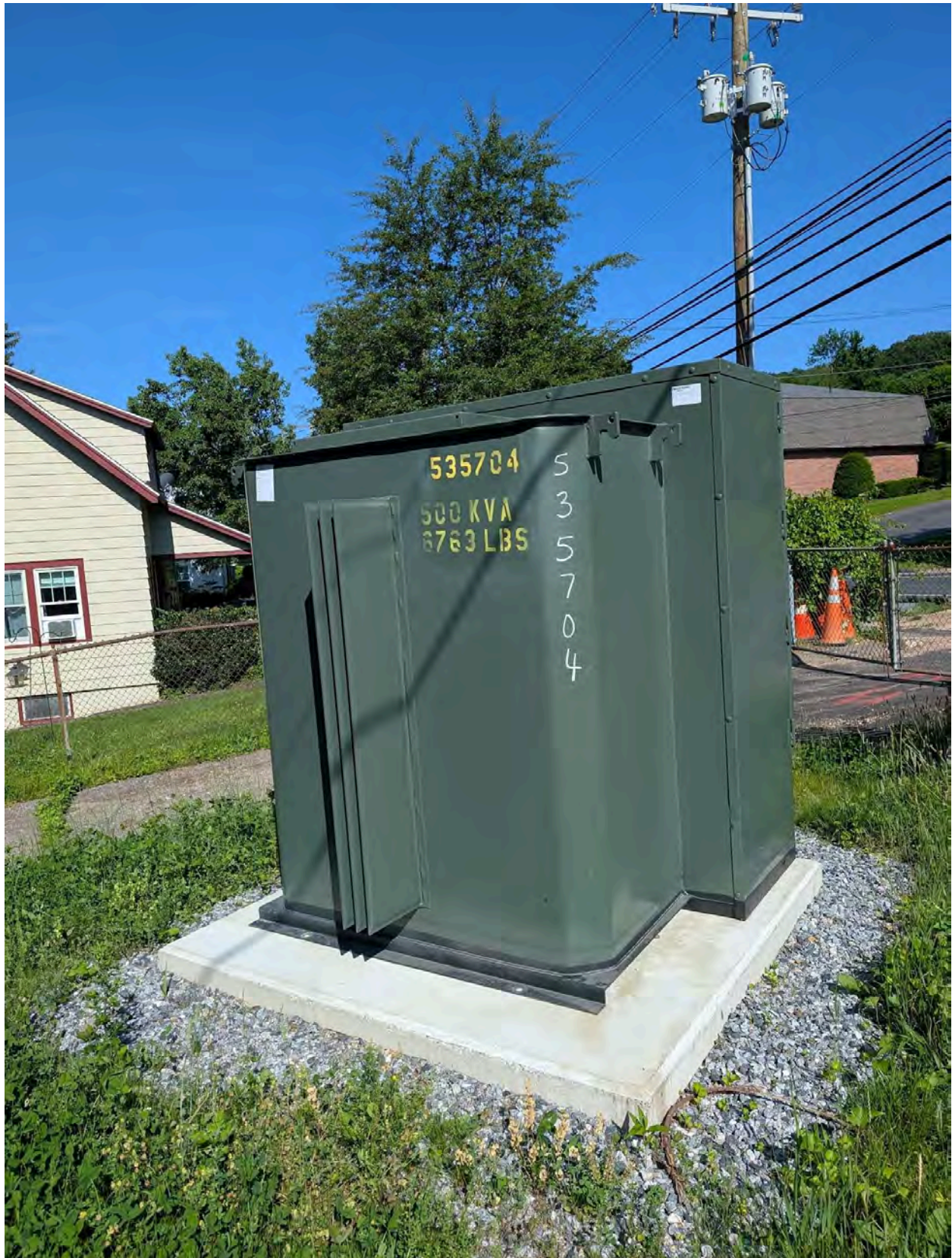
Exhibit 3.2 - M.M Generali Photos of Existing Transformer
