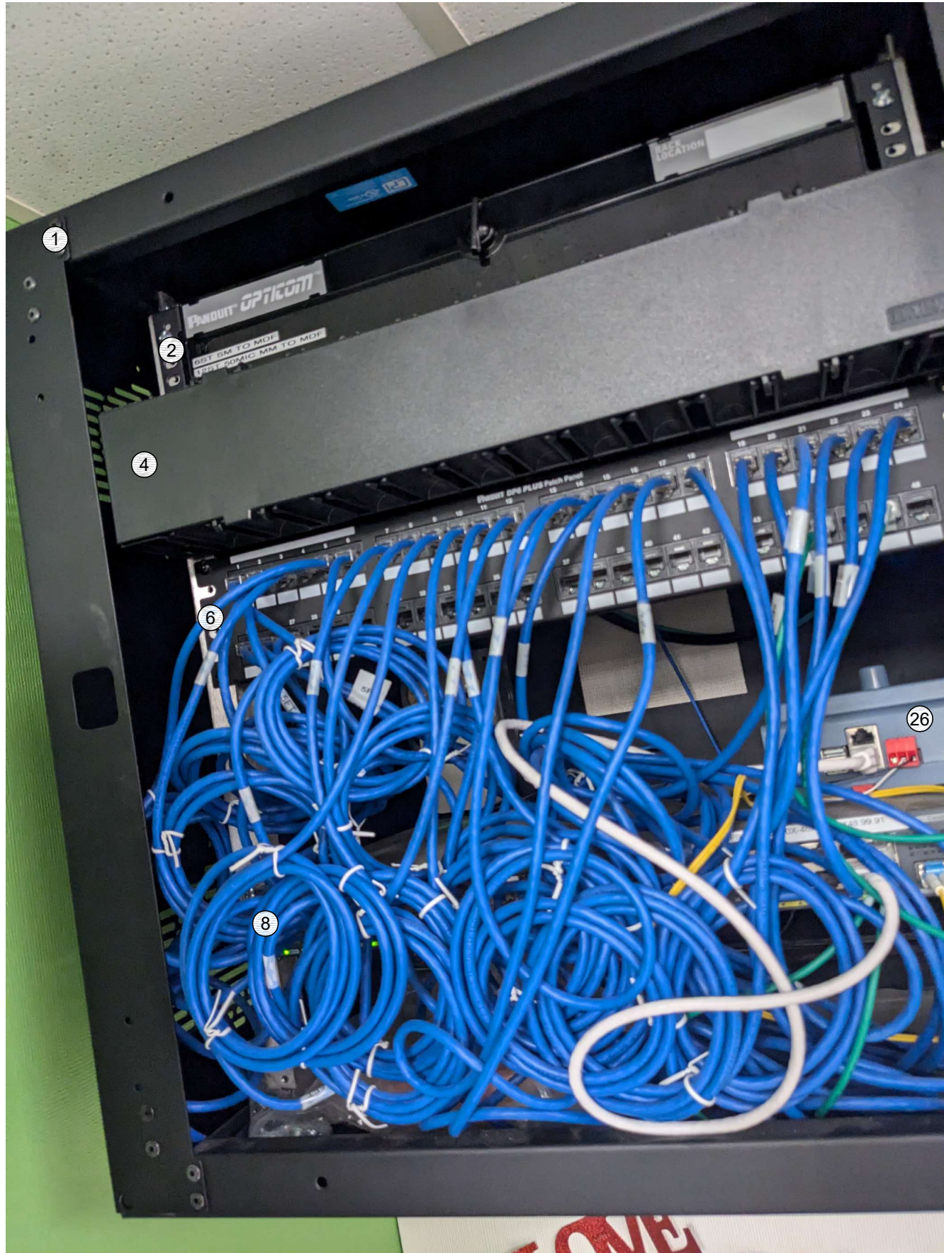
RACK - EXISTING CONDITION SCALE: NONE
