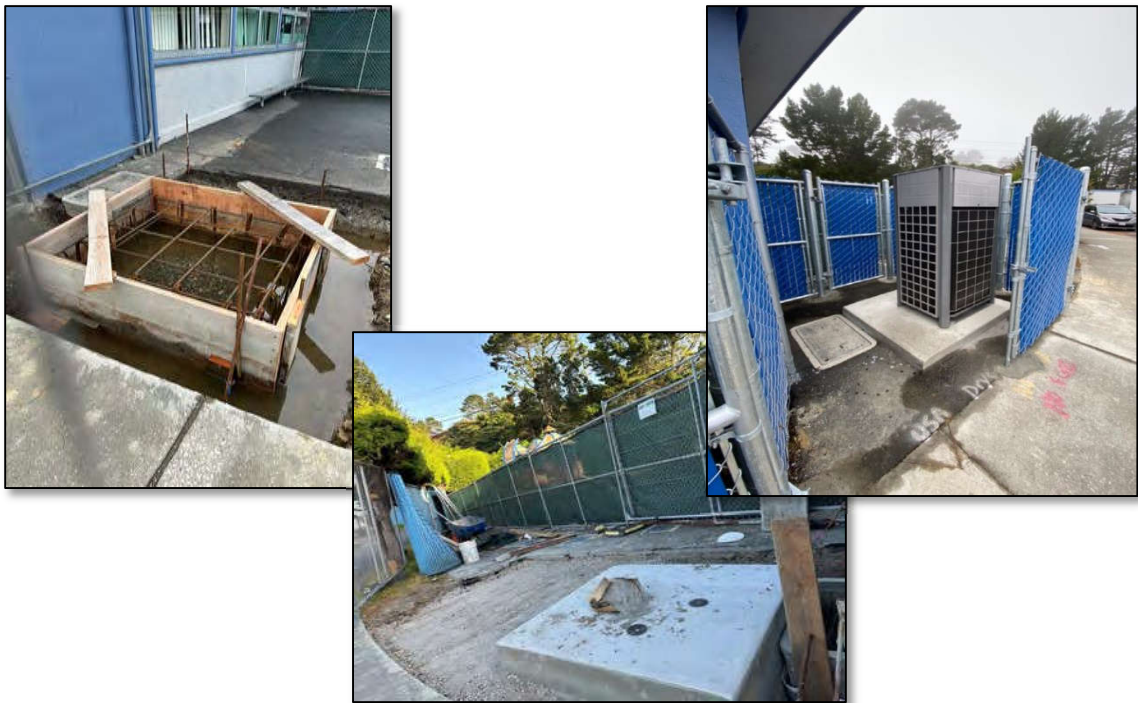
Equipment Pad for Unit
