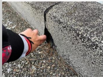
Photo 14 Theater Hole in flashings at seams
