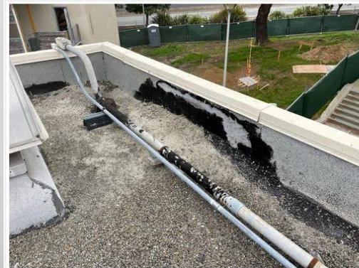
Photo 20 Theater Previous repairs done with mastic.
