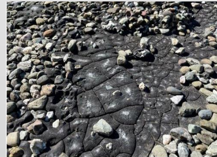
Cracks in membrane.
