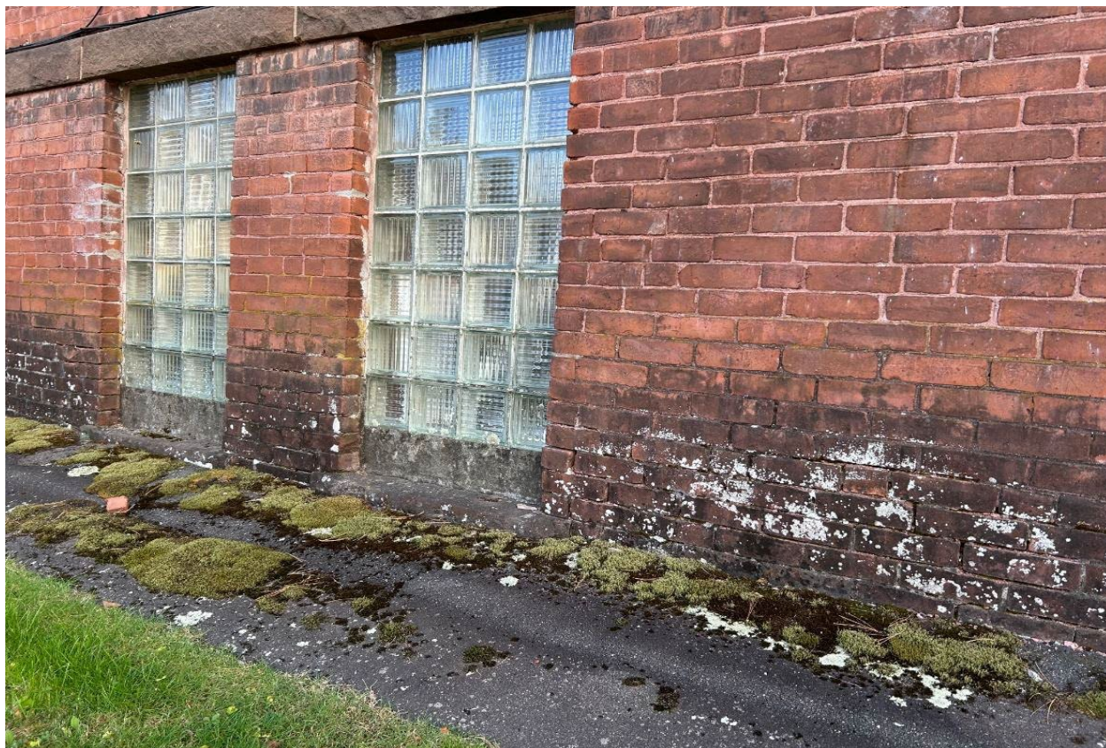
West elevation brick and mortar deterioration
