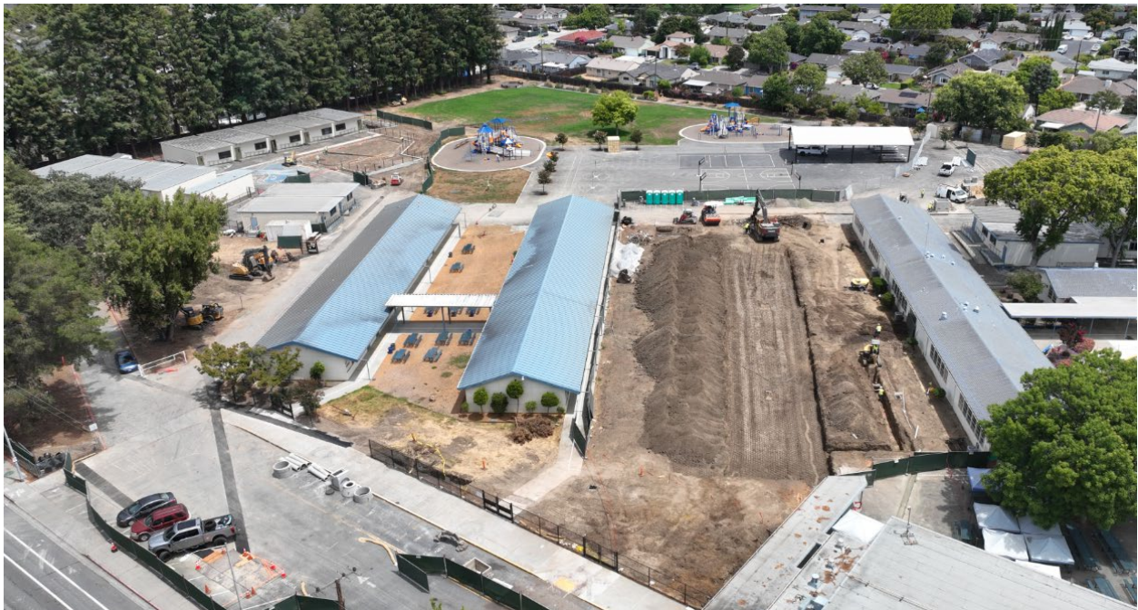
Aerial view on July 22, 2025. The building pad is being constructed for the new multipurpose building. Pending testing, the soil will be used at the New Laurelwood Elementary School site. The new preschool playground is in the upper left corner of the photo. A new underground storm water retention structure and new connection to Saratoga Avenue can be seen on the left.
