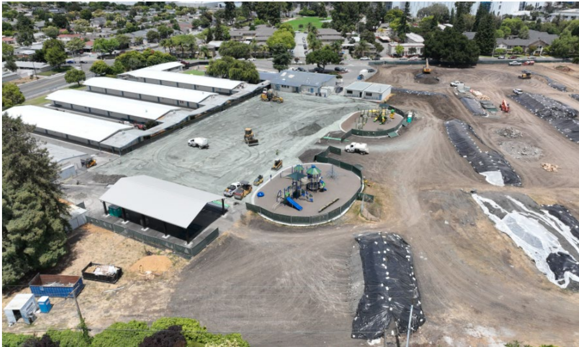
Aerial view looking northwest on July 22, 2025. Roofs are ready for steel panels. Playground is ready for asphalt paving. Contaminated soil is stockpiled in the field for testing and off-site disposal.
