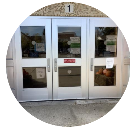
Access Controls Upgrade
