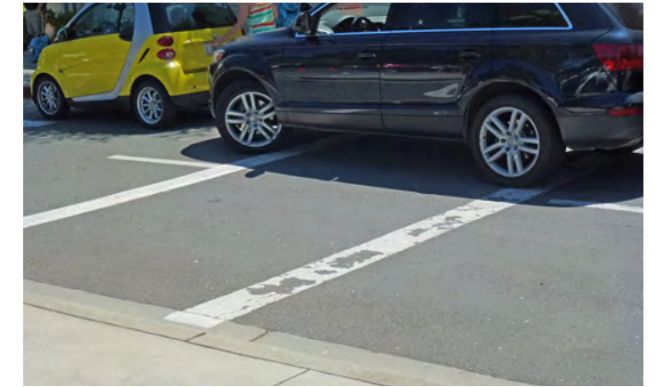
Crosswalk within school parking lot; parking violation and lack of curb ramp.
