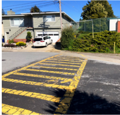
Figure 8. Fading high-visibility crosswalk across Avalon Dr.
