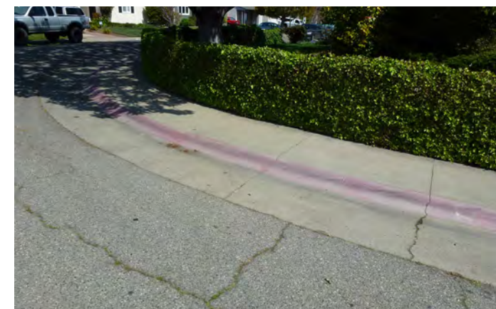
Curb paint needs restriping and there may be other visibility challenges on W. Grant Place.
