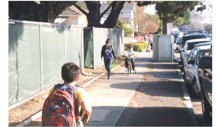
An asphalt paved area adjacent to the concrete sidewalk is not in good condition, but may help to increase pedestrian space.
