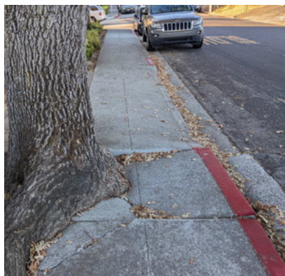
Figure 11. Sidewalk in disrepair on Clifford Ave.
