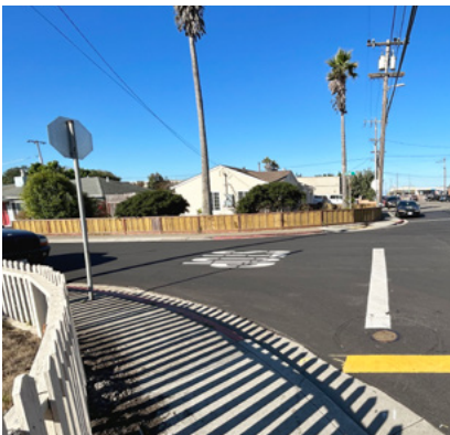
Figure 10. Missing crosswalk across Johnson Ave at Manor Dr.
