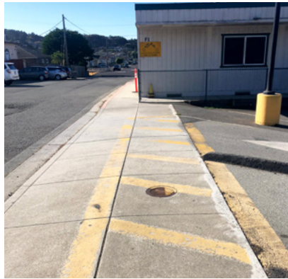
Figure 5. Fading crosswalk at the dead-end on Edgemar Ave.
