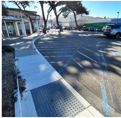
Figure 2. Fading pavement markings inside school parking lot.
