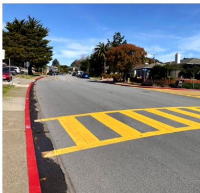
Figure 1. Missing curb ramps at Helen Dr/Mosswood Ln
