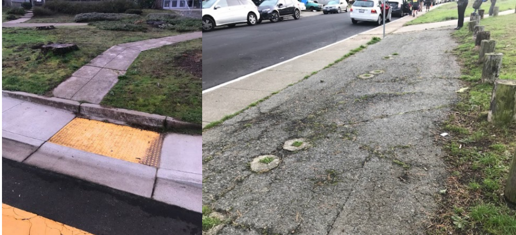
Left: Old curb at school property line creates an accessibility barrier. Right: Uneven, degrading asphalt pavement adjacent to sidewalk between the drop off loop and school entry path along school frontage.
