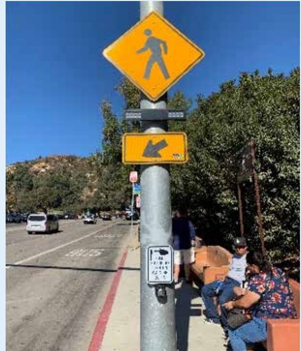
Rectangular Rapid Flashing Beacons (RRFBs)
