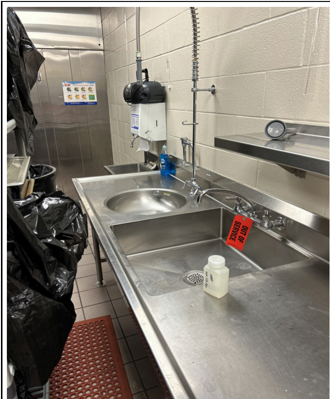
6/27/2024 - 1000-148 - South Valley - 004677- Kitchen East Wall- Next to Fridge
