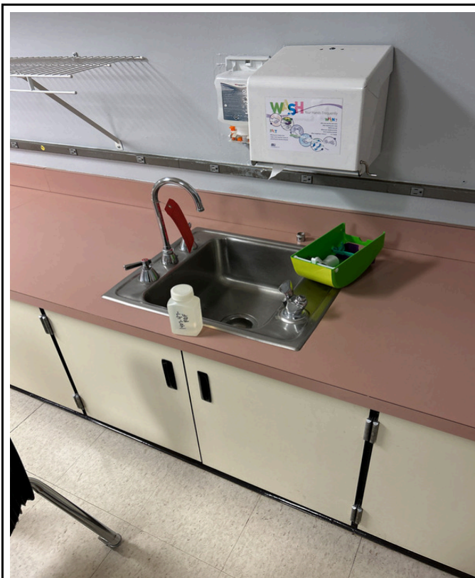
6/28/2024 - 1407-47 - Lewis and Clark - 001277F-Room 48-South Sink
