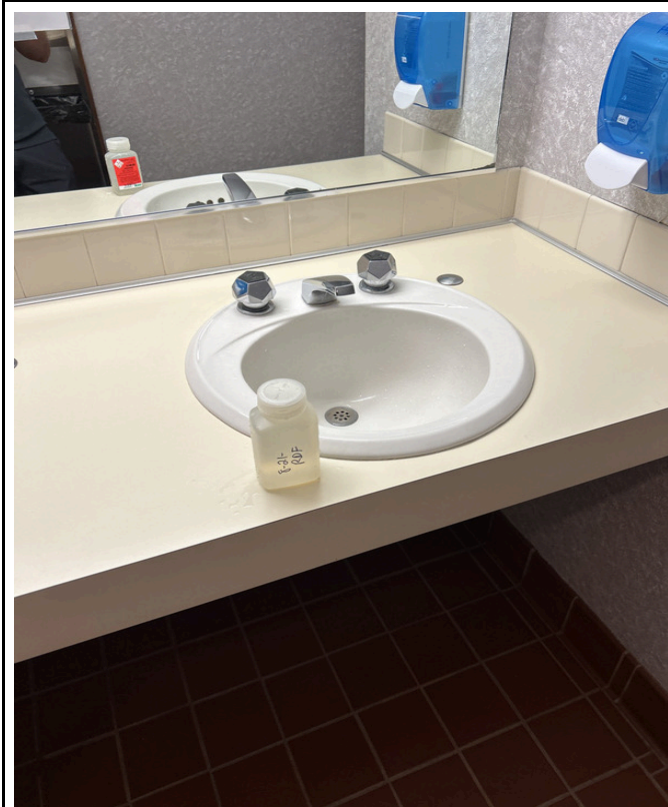
6/28/2024 - 8-21 - District Administration Center - 004551-By Elevator 2nd Floor-Boys-Right
