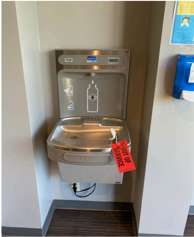
9/4/2024 - 8-2 - District Administration Center - 004563F-By Elevator 4th Floor
