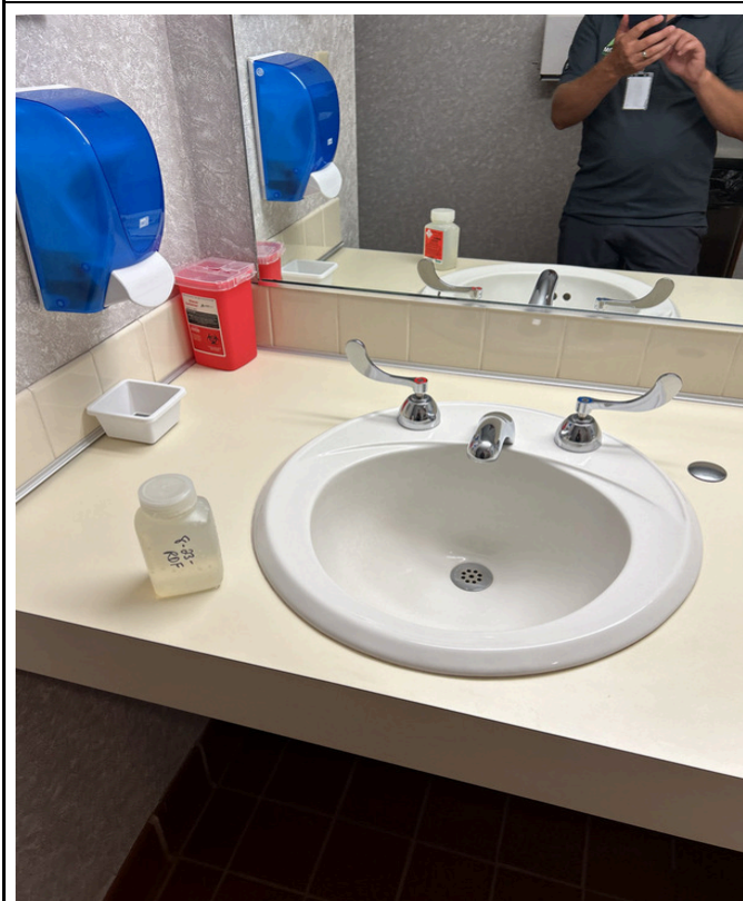
6/28/2024 - 8-23 - District Administration Center - 004553-By Elevator 2nd Floor-Girls-Left
